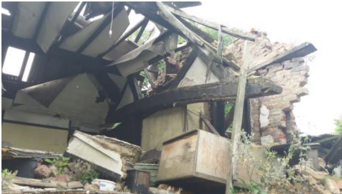
13: NORTH ELEVATION. CENTRAL BAY OF MAIN RANGE, ADJACENT TO DEMOLISHED PORTION OF BUILDING. UNSUPPORTED ROOF STRUCTURE. TIMBER ROOF TRUSS APPEARS LARGELY INTACT. FIRST FLOOR IS IN SITU.
