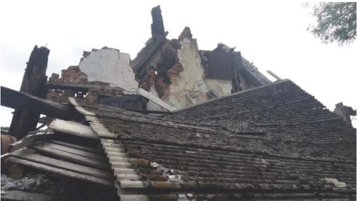
11: WEST ELEVATION. EXTENSIVE COLLAPSE; NOTE INTERNAL BRICK WALL AND CHIMNEY.
