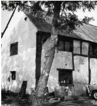
1970a: WEST END OF THE MAIN RANGE, NOW LARGELY COLLAPSED. NOTE THE ROOF COVERINGS, APPARENTLY THOSE STILL PRESENT.
