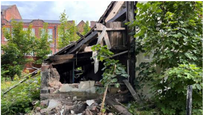
04: SOUTH ELEVATION. WEST END OF MAIN RANGE. ROOF AND FIRST FLOOR ALMOST TOTALLY COLLAPSED.
