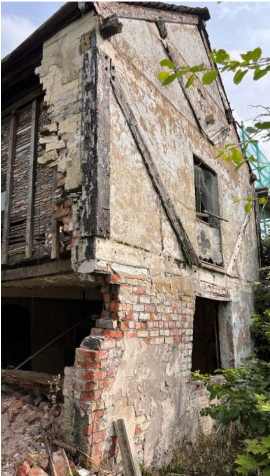
05: SOUTH ELEVATION. GABLE WALL OF CROSSWING. BRICK WALL AT GROUND FLOOR LEVEL IS SIGNIFICANTLY OUT OF PLUMB. NOTE GIRDING RAIL, WITH TENON FOR NOW-REMOVED CORNER POST.
