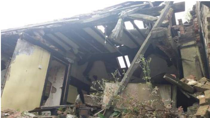
12: NORTH ELEVATION. CENTRAL BAY OF MAIN RANGE, ADJACENT TO DEMOLISHED PORTION OF BUILDING. LOOKING INTO ROOM F6. UNSUPPORTED ROOF STRUCTURE.
