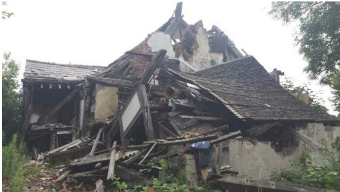
10: WEST ELEVATION. GENERAL VIEW. EXTENSIVE COLLAPSE AT THE WESTERN END OF THE MAIN RANGE.
