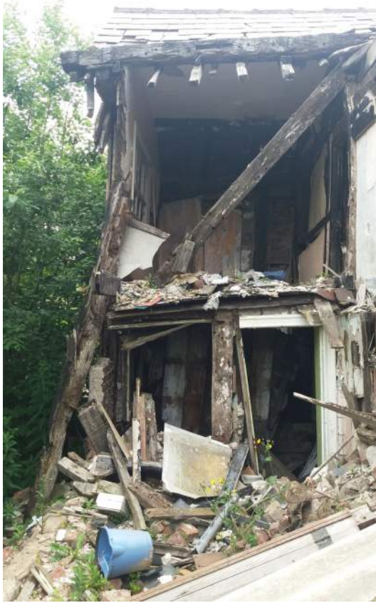
16: NORTH ELEVATION. SIDE OF PROJECTION FROM MAIN RANGE, ADJACENT TO DEMOLISHED PORTION OF BUILDING. FIRST FLOOR AND ROOF ARE LARGELY INTACT; CORNER POST OF PROJECTION HAS BEEN REMOVED.
