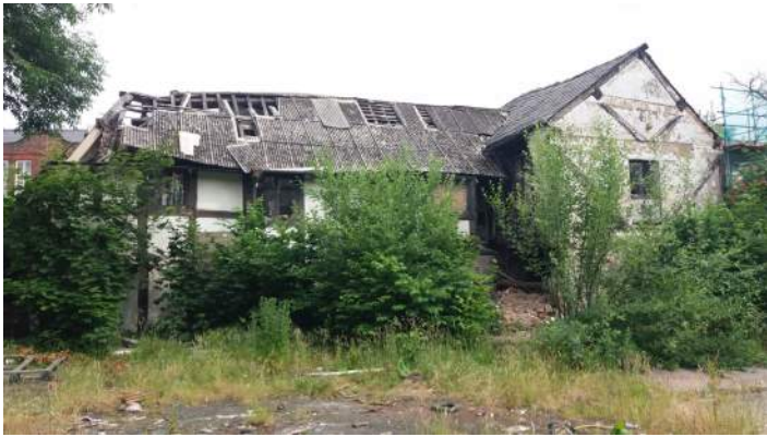
03: SOUTH ELEVATION. GENERAL VIEW. COLLAPSED PORTION OF MAIN RANGE IS AT THE LEFT OF FRAME.
