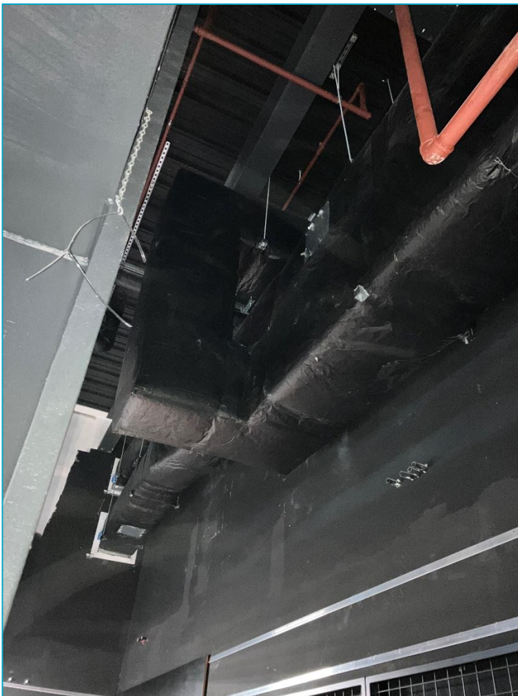
Figure 6 – Installed ductwork, including dense lagging
