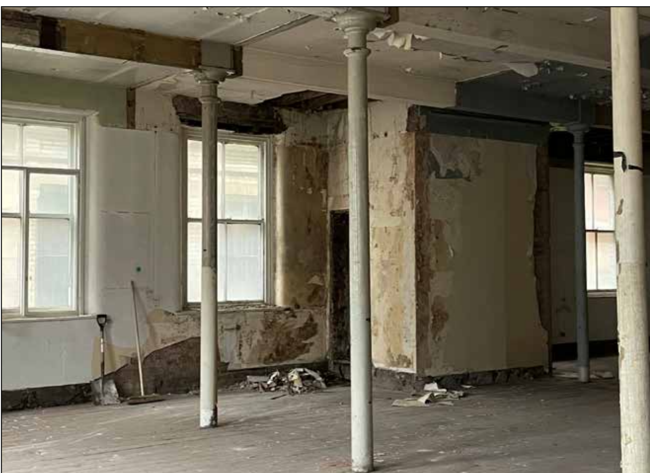
Image 48: Photograph showing housing for former hoist, damaged and with non-original opening inserted.
