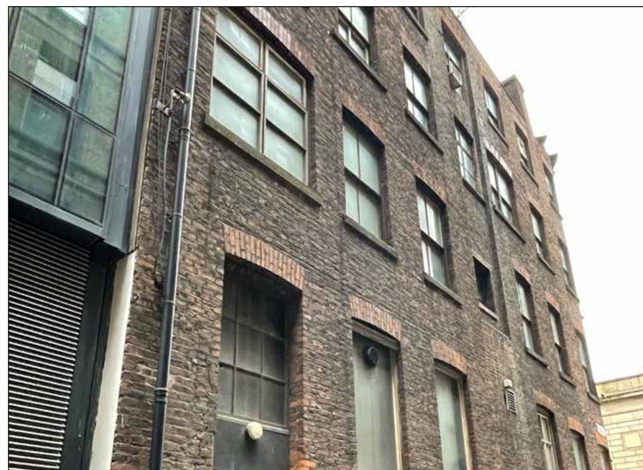
Image 16: Photograph showing one over one sliding sash windows to Mosley/Princess St. corner, with non-original secondary glazing.
