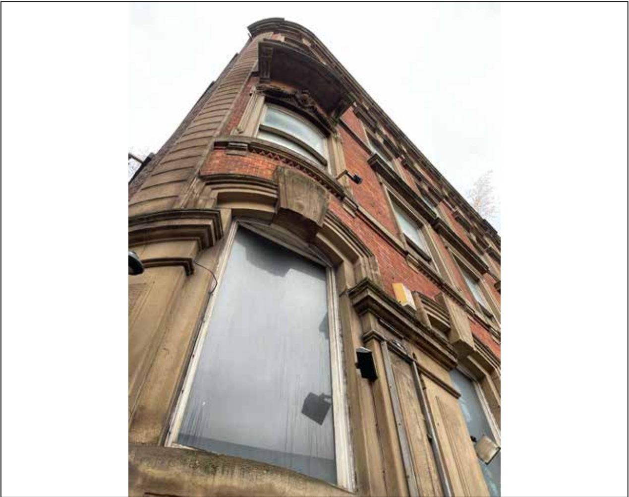
Image 28: Detail of corner of Princess/Back George St. with original rounded windows and later flat replacement versions.
