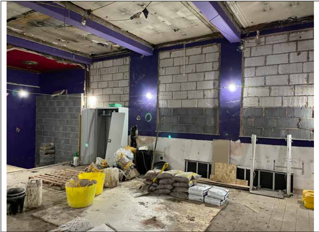
Image 50: Blocked up openings to ground floor unit along Princess St.
