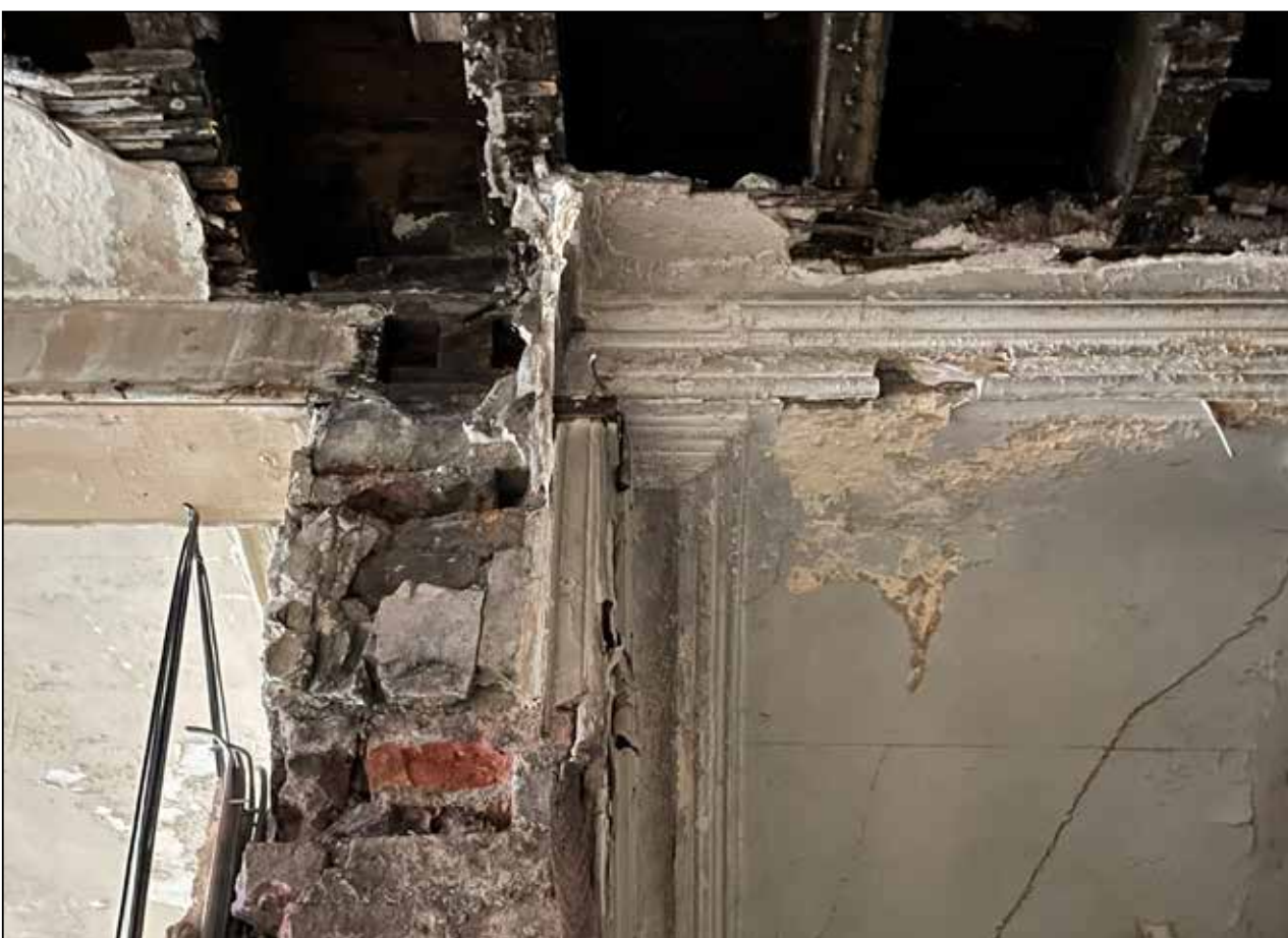
Image 49: First floor, damaged cornicing and evidence of lath and plaster finishes.
