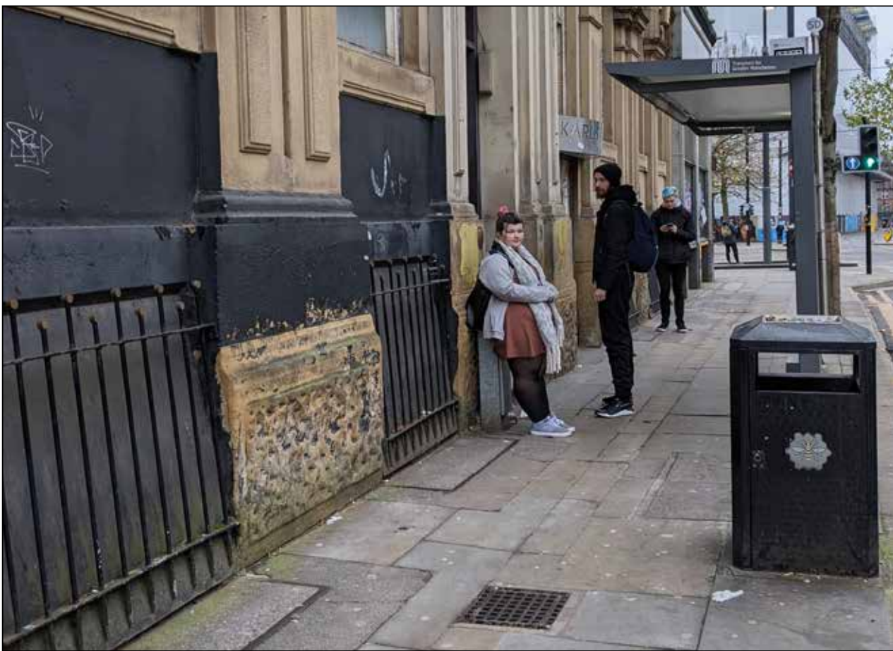
Image 67: Photograph showing existing street scape with boarded windows, over-painted stone and graffiti.
