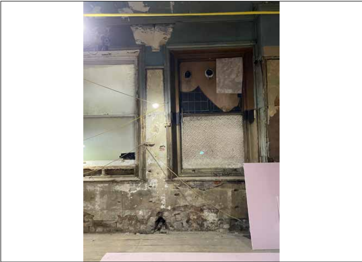
Image 52: Blocked up windows to lightwell on ground floor.
