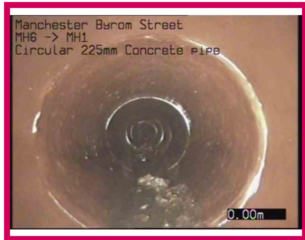
2, 00:00:05, 0.00 m Settled deposits, fine, 5% cross-sectional area loss
