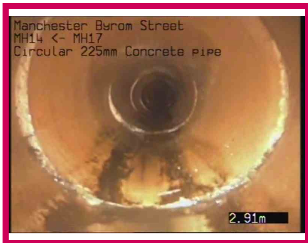
3, 00:00:23, 2.91 m Crack, longitudinal at joint at 8 o'clock
