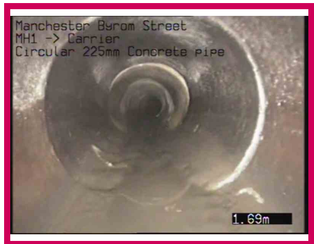
4, 00:00:15, 1.69 m Settled deposits, fine, 10% cross-sectional area loss
