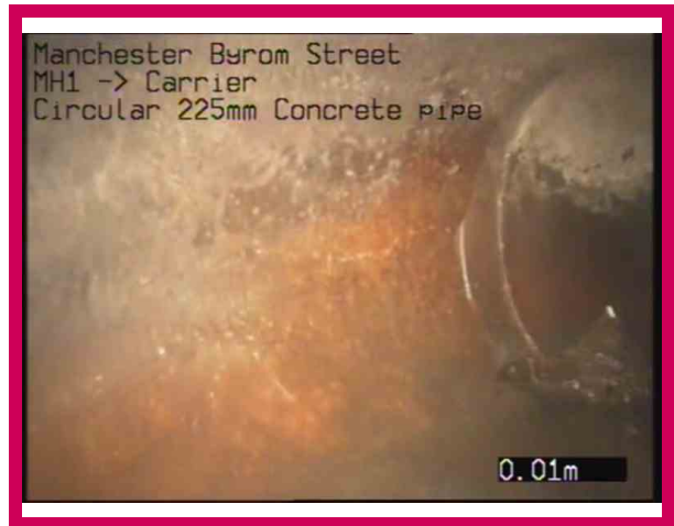
2, 00:00:07, 0.01 m Settled deposits, coarse at joint, 5% cross-sectional area loss
