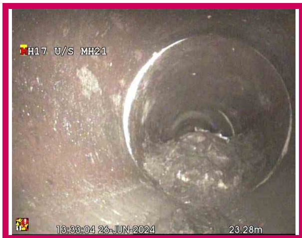
3, 00:02:23, 23.28 m Settled deposits, fine, 10% cross-sectional area loss, finish
