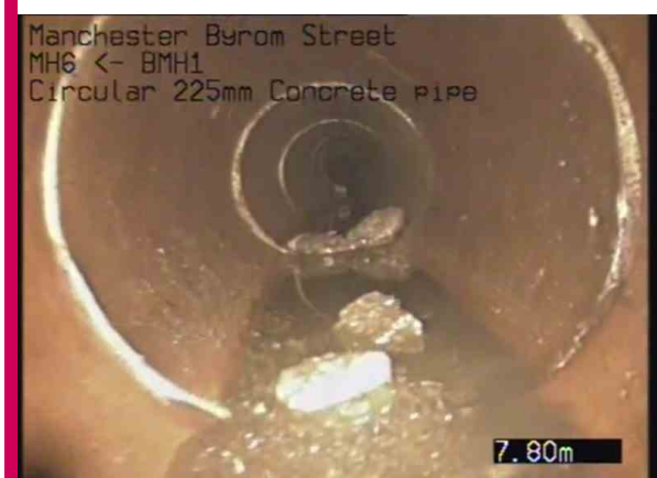
6, 00:00:30, 7.80 m Settled deposits, fine, 5% cross-sectional area loss
