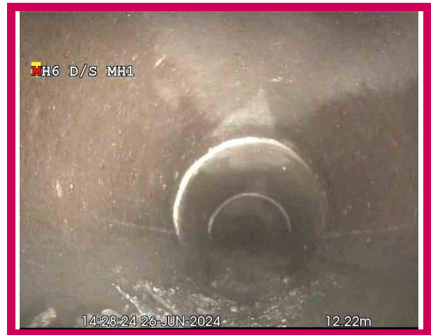
2, 00:01:14, 12.22 m Settled deposits, fine, 10% cross-sectional area loss
