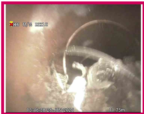
3, 00:01:03, 11.86 m Settled deposits, fine, 50% cross-sectional area loss
