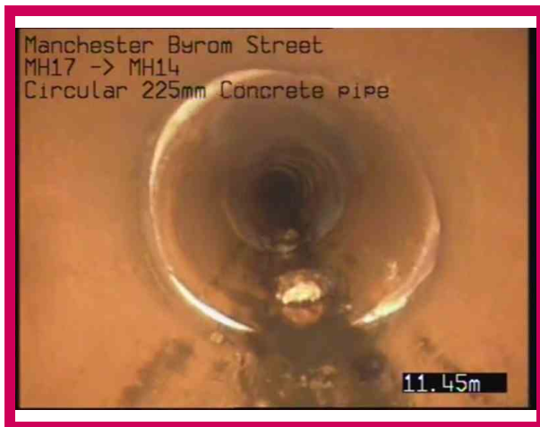
3, 00:00:54, 11.57 m Settled deposits, coarse, 5% cross-sectional area loss
