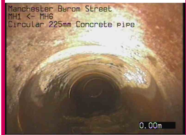
2, 00:00:06, 0.00 m Settled deposits, fine, 20% cross-sectional area loss
