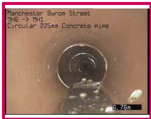
6, 00:00:33, 6.76 m Settled deposits, fine, 5% cross-sectional area loss
