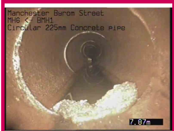
8, 00:00:33, 7.87 m Settled deposits, coarse at joint, 10% cross-sectional area loss
