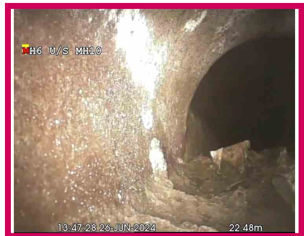
4, 00:01:52, 22.54 m Settled deposits, hard or compacted, 10% cross-sectional area loss
