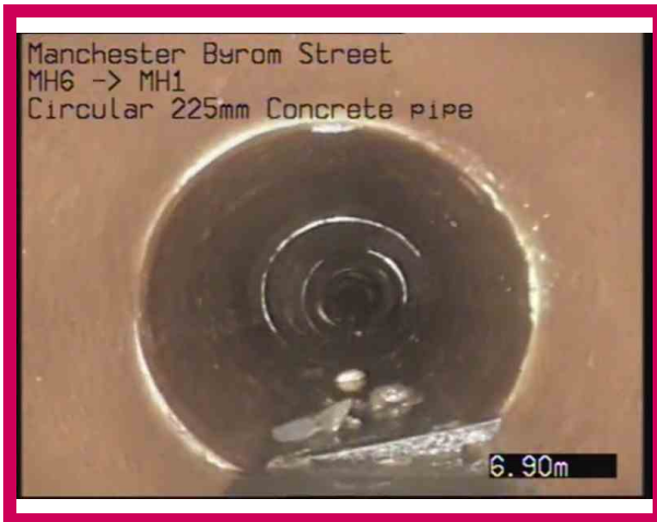
7, 00:00:35, 6.90 m Settled deposits, coarse at joint, 10% cross-sectional area loss
