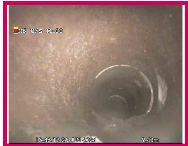
2, 00:00:37, 9.43 m Settled deposits, fine, 10% cross-sectional area loss
