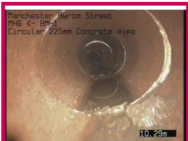
10, 00:00:49, 10.29 m Settled deposits, fine at joint, 5% cross-sectional area loss
