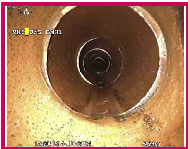
3, 00:00:55, 8.69 m Junction at 3 o'clock, diameter: 150mm
