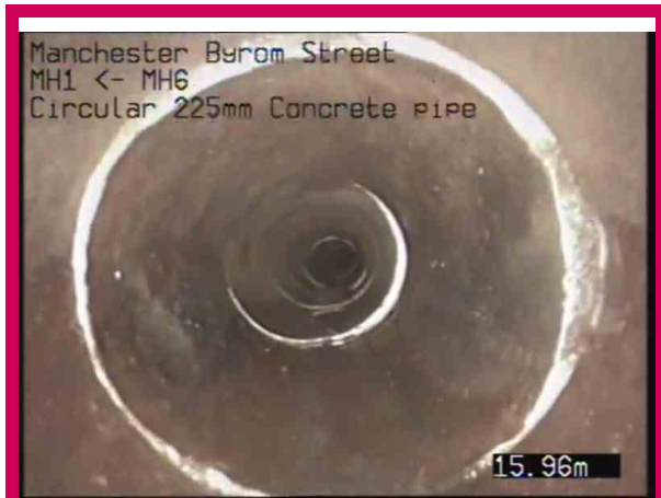
10, 00:01:16, 15.96 m Surface damage, spalling from 2 o'clock to 4 o'clock
