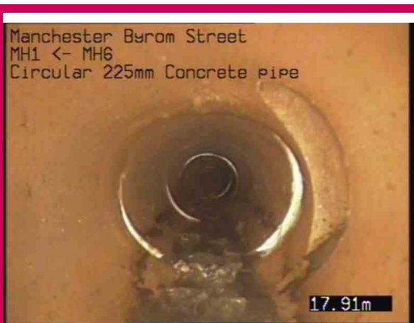
11, 00:01:23, 17.91 m Settled deposits, fine, 5% cross-sectional area loss
