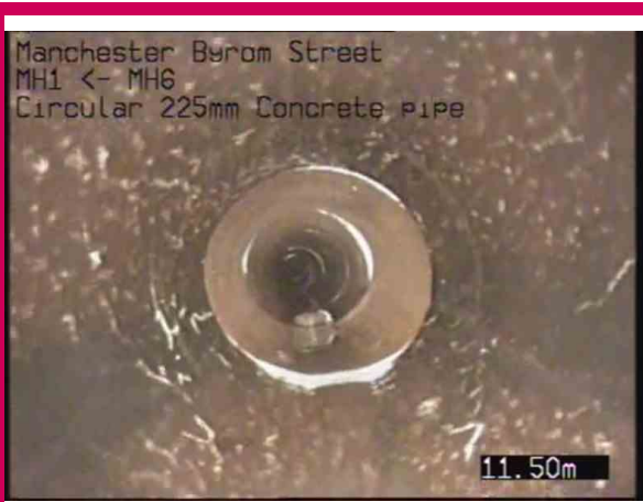
7, 00:00:52, 11.50 m Cracks, multiple from 12 o'clock to 2 o'clock
