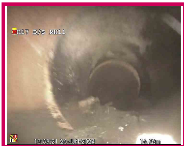
3, 00:00:52, 16.89 m Settled deposits, fine, 10% cross-sectional area loss
