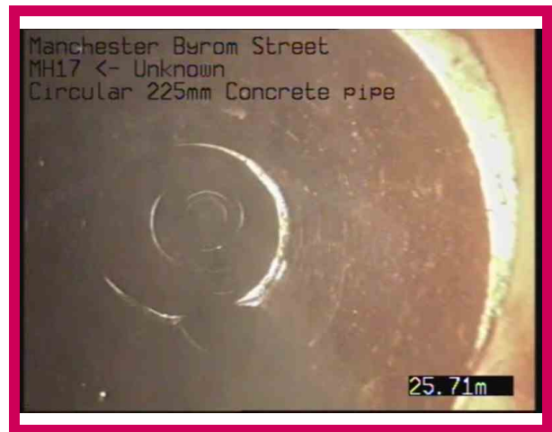
8, 00:02:10, 25.52 m Joint displaced, medium
