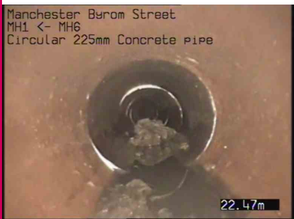
13, 00:01:45, 22.47 m Settled deposits, fine, 10% cross-sectional area loss
