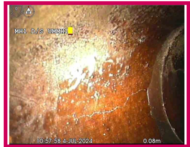
2, 00:00:05, 0.04 m Crack, longitudinal at joint at 9 o'clock
