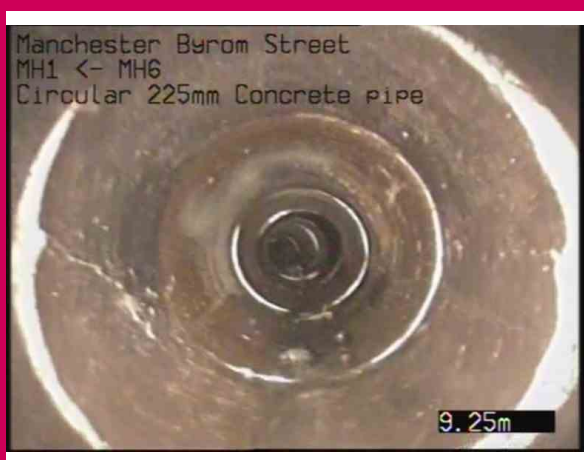
5, 00:00:45, 9.25 m Crack, longitudinal at joint at 3 o'clock
