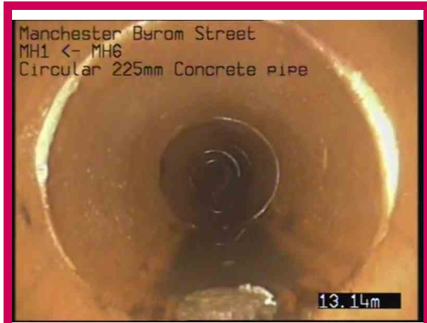
8, 00:00:57, 13.14 m Settled deposits, coarse at joint, 5% cross-sectional area loss
