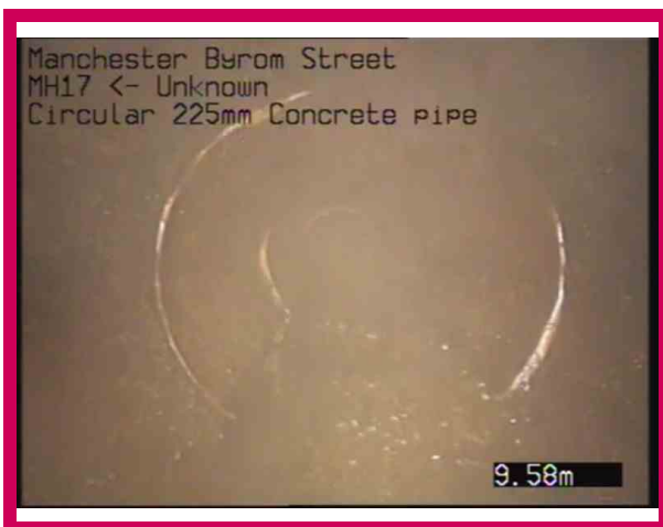
5, 00:00:47, 11.14 m Settled deposits, fine, 15% cross-sectional area loss, start
