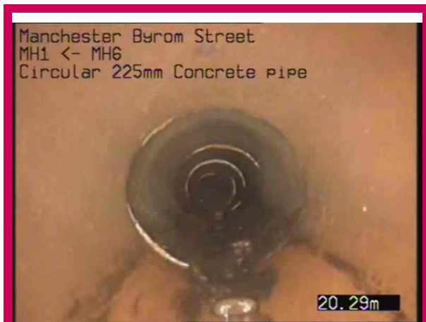
12, 00:01:34, 20.29 m Settled deposits, coarse, 5% cross-sectional area loss
