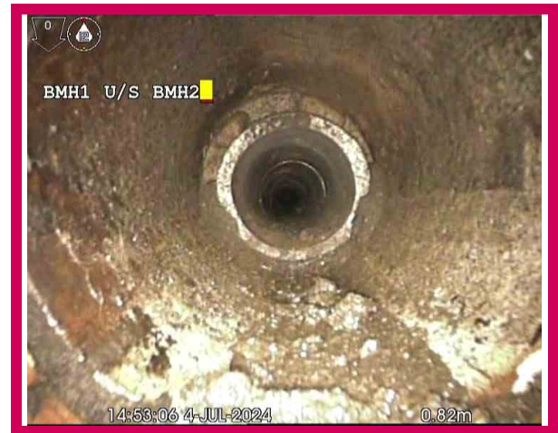
2, 00:00:07, 0.76 m Settled deposits, fine, 10% cross-sectional area loss
