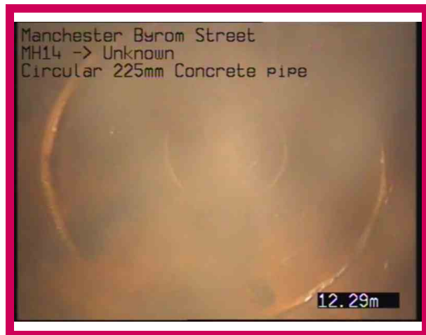
4, 00:00:55, 12.29 m Settled deposits, fine, 10% cross-sectional area loss, finish
