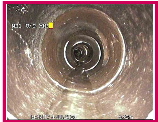
2, 00:00:47, 6.92 m Fracture, longitudinal at 9 o'clock
