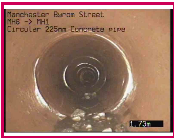
3, 00:00:13, 1.73 m Settled deposits, coarse, 5% cross-sectional area loss
