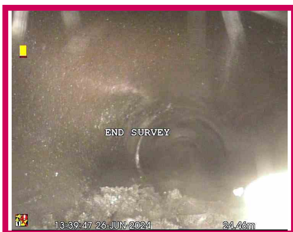
5, 00:02:17, 24.47 m Survey abandoned, Unable to survey further due to debris in line.
