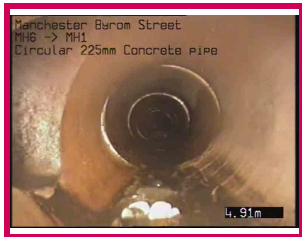
4, 00:00:26, 4.91 m Settled deposits, coarse, 5% cross-sectional area loss
