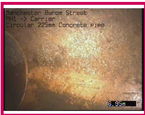
5, 00:00:48, 6.91 m Finish node, other special chamber, reference: Carrier, Line drops into carrier
