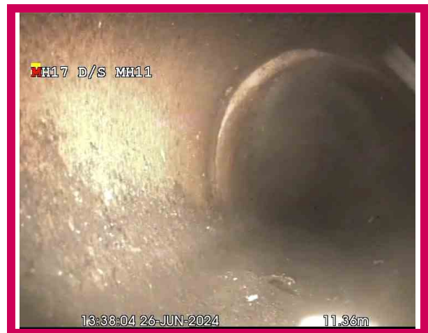
2, 00:00:35, 11.36 m Settled deposits, hard or compacted, 10% cross-sectional area loss
