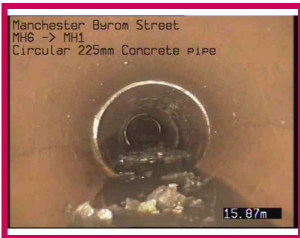
9, 00:01:11, 15.87 m Settled deposits, coarse, 15% cross-sectional area loss
