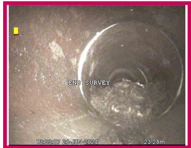
2, 00:02:29, 23.28 m Survey abandoned, Unable to survey further due to debris in line.
