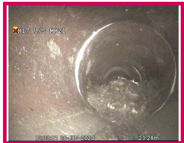
4, 00:02:23, 23.28 m Settled deposits, hard or compacted, 30% cross-sectional area loss
