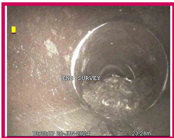
5, 00:02:29, 23.28 m Survey abandoned, Unable to survey further due to debris in line.
