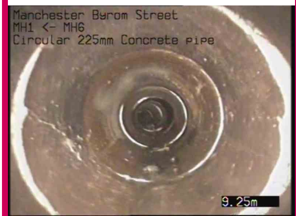
4, 00:00:45, 9.25 m Crack, longitudinal at joint at 9 o'clock
