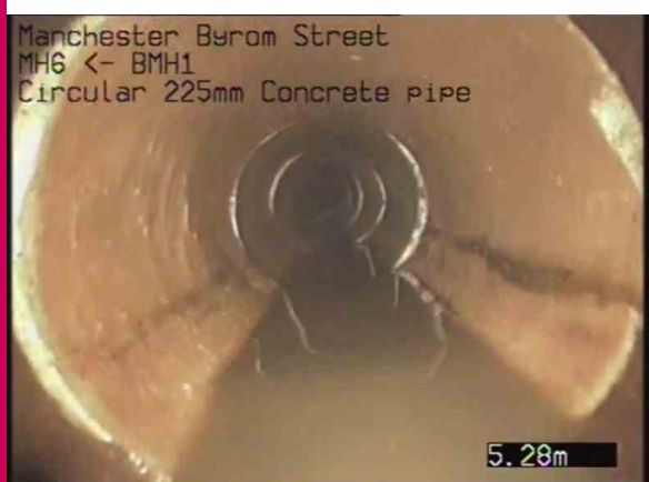
5, 00:00:20, 5.28 m Surface damage, spalling from 2 o'clock to 3 o'clock
