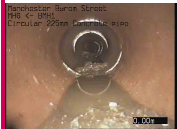
2, 00:00:04, 0.00 m Settled deposits, fine, 10% cross-sectional area loss
