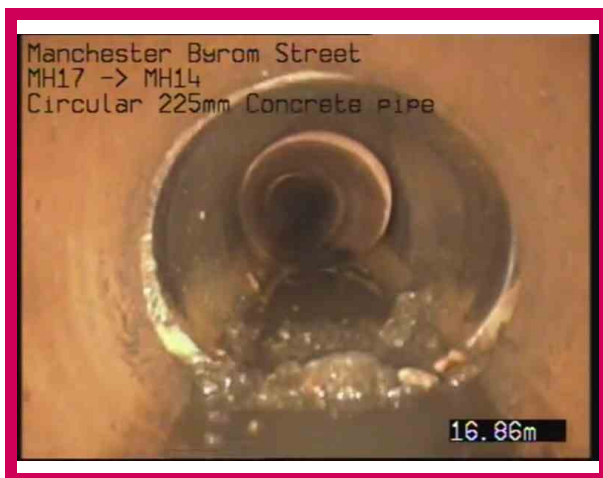
5, 00:01:19, 16.86 m Settled deposits, coarse, 10% cross-sectional area loss
