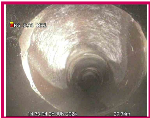
3, 00:05:53, 29.34 m Survey abandoned, Unable to survey due to debris in line.
