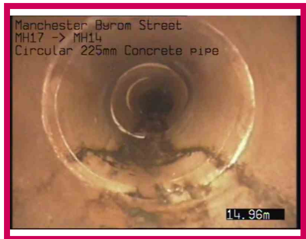
4, 00:01:11, 14.96 m Crack, circumferential at joint from 12 o'clock to 12 o'clock
