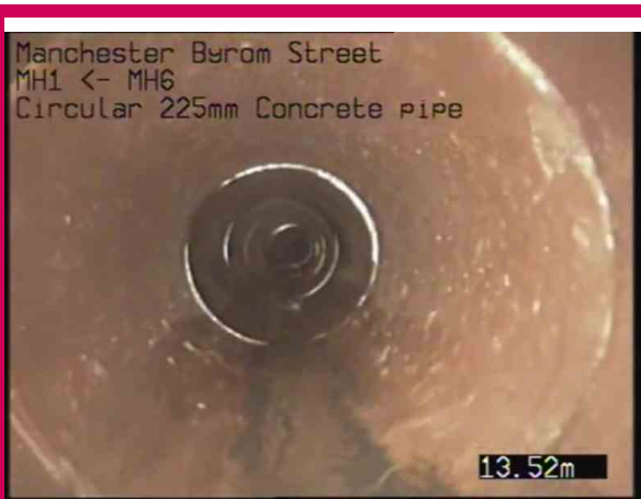
9, 00:01:03, 13.52 m Surface damage, spalling at 2 o'clock
