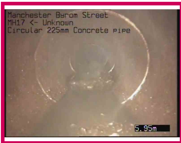
3, 00:00:33, 5.95 m Settled deposits, fine, 10% cross-sectional area loss
