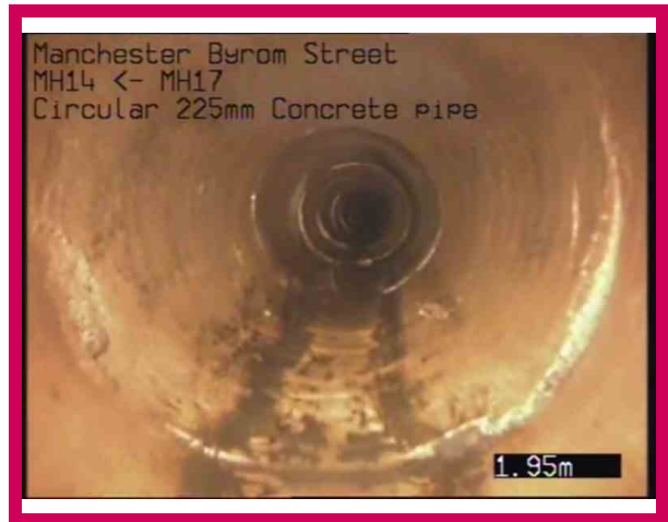
2, 00:00:16, 1.95 m Surface damage, spalling from 8 o'clock to 9 o'clock
