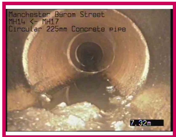
4, 00:00:47, 8.55 m Survey abandoned, Unable to survey past connection dropping debris while jetting. No access into line to flush or jet.
