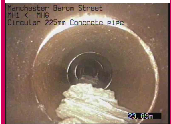
14, 00:01:55, 23.89 m Settled deposits, hard or compacted at joint, 30% cross-sectional area loss
