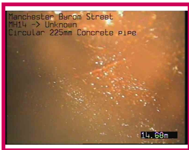
5, 00:01:09, 14.69 m Finish node, other special chamber, reference: Unknown, Line goes left into carrier
