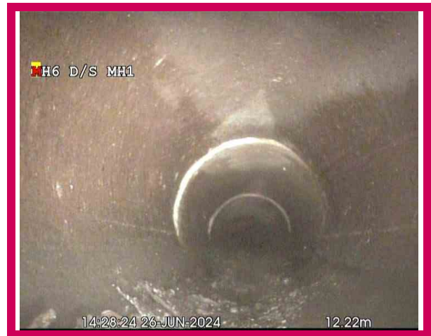
2, 00:01:14, 12.22 m Settled deposits, fine, 10% cross-sectional area loss
