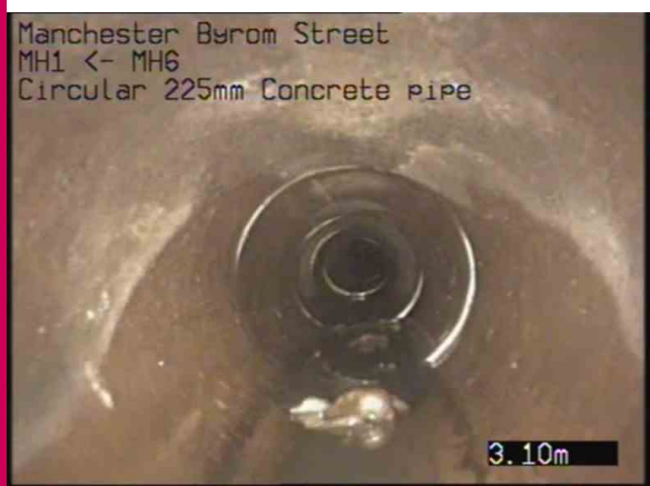
3, 00:00:22, 3.10 m Settled deposits, coarse, 5% cross-sectional area loss
