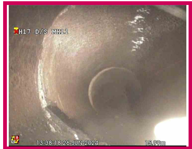
2, 00:00:48, 15.99 m Attached deposits, encrustation at joint from 6 o'clock to 8 o'clock, 5% cross-sectional area loss
