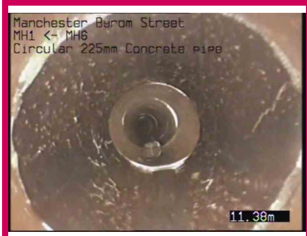
6, 00:00:52, 11.38 m Crack, longitudinal at joint at 2 o'clock
