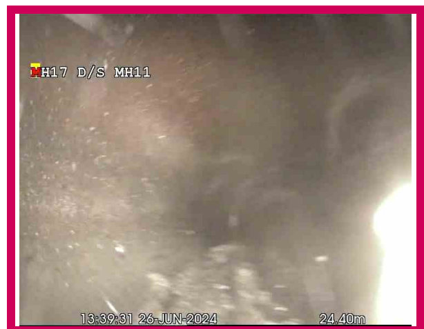
4, 00:02:02, 24.40 m Settled deposits, fine, 10% cross-sectional area loss
