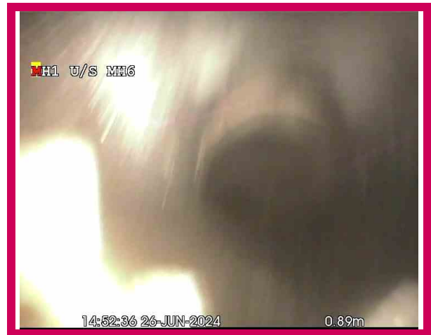
2, 00:00:12, 0.89 m Settled deposits, fine, 10% cross-sectional area loss
