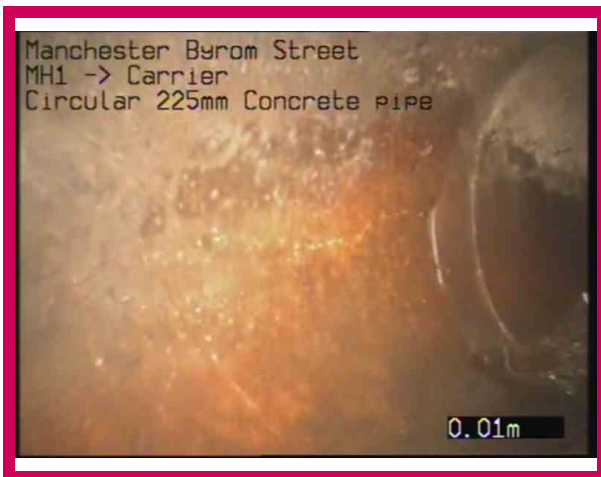
3, 00:00:07, 0.01 m Crack, longitudinal at joint at 9 o'clock
