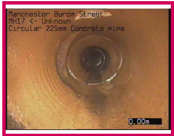
2, 00:00:02, 0.00 m Surface damage, spalling at 12 o'clock
