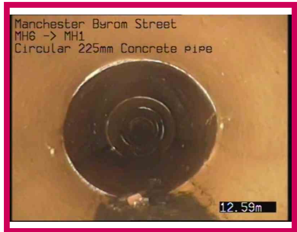
8, 00:00:56, 12.59 m Settled deposits, coarse, 5% cross-sectional area loss
