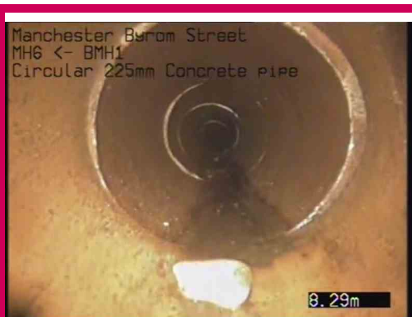
9, 00:00:41, 10.29 m Settled deposits, coarse, 10% cross-sectional area loss
