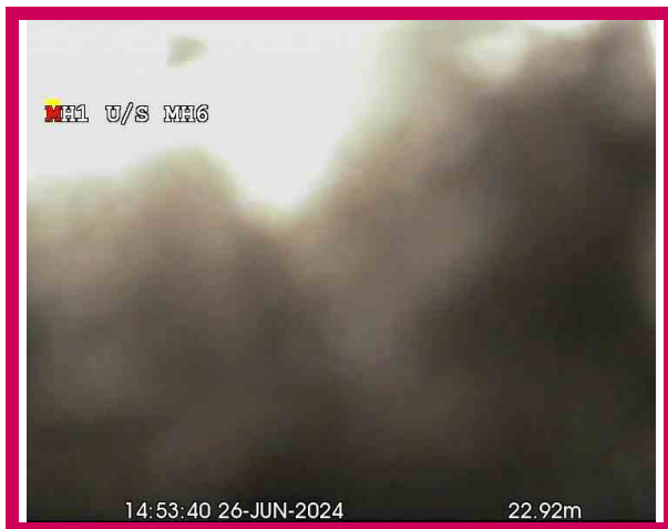
3, 00:01:16, 22.92 m Settled deposits, fine, 40% cross-sectional area loss
