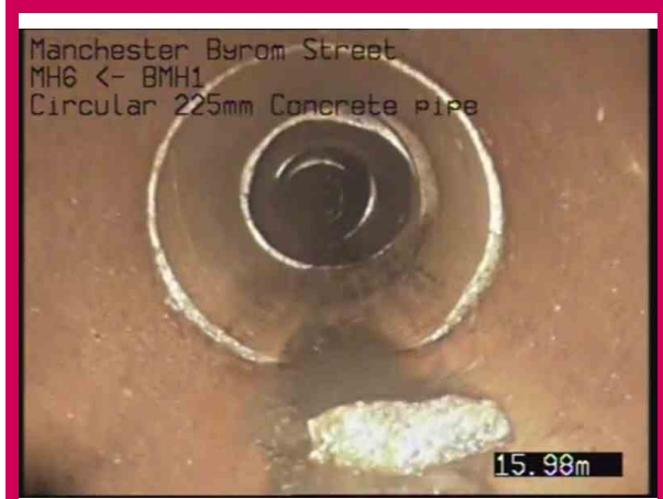
14, 00:01:16, 15.98 m Settled deposits, coarse, 5% cross-sectional area loss
