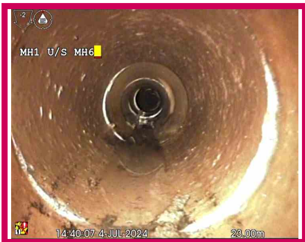
3, 00:02:36, 23.00 m Settled deposits, fine, 5% cross-sectional area loss
