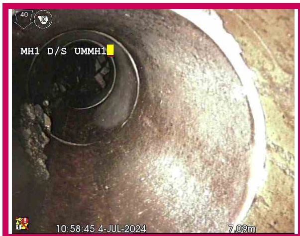
3, 00:00:52, 7.09 m Finish node, other special chamber, reference: UMMH1, Carrier line to UMMH1.
