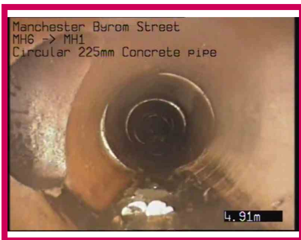
5, 00:00:25, 4.92 m Settled deposits, fine, 5% cross-sectional area loss
