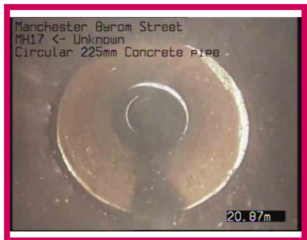
6, 00:01:36, 20.87 m Surface damage, spalling from 12 o'clock to 2 o'clock
