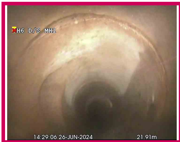
3, 00:01:55, 21.39 m Settled deposits, fine, 10% cross-sectional area loss
