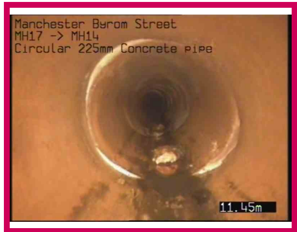
2, 00:00:53, 11.45 m Deformed drain or sewer, 5%
