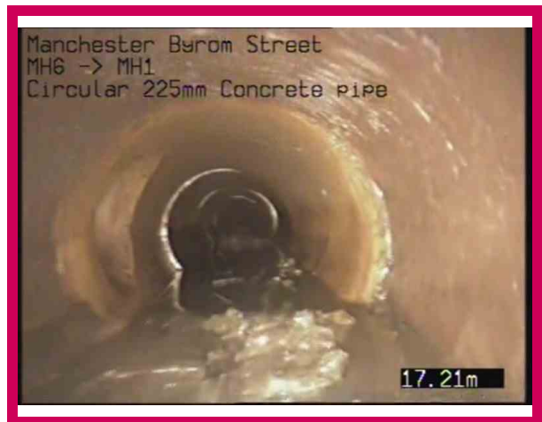
10, 00:01:15, 17.55 m Settled deposits, coarse, 20% cross-sectional area loss
