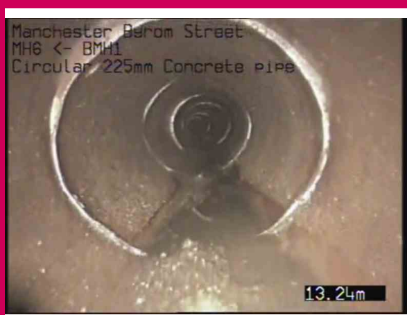
13, 00:01:03, 13.24 m Settled deposits, fine, 5% cross-sectional area loss
