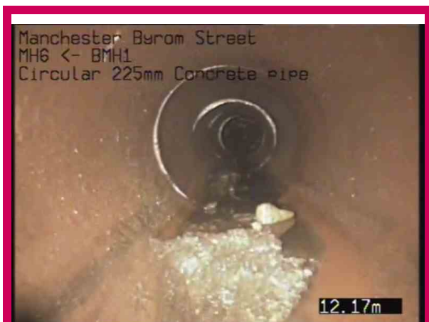
12, 00:00:59, 12.17 m Settled deposits, fine, 10% cross-sectional area loss
