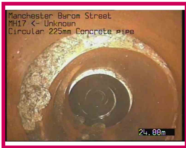
7, 00:02:00, 24.81 m Joint displaced, medium
