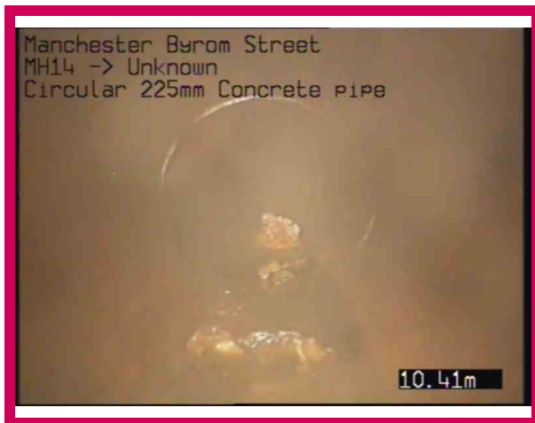
3, 00:00:46, 10.48 m Settled deposits, coarse, 10% cross-sectional area loss
