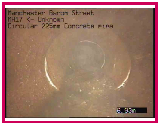
4, 00:00:36, 7.07 m Settled deposits, fine, 20% cross-sectional area loss
