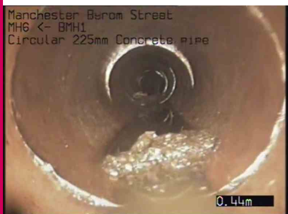
3, 00:00:06, 0.44 m Settled deposits, fine, 10% cross-sectional area loss
