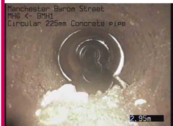
4, 00:00:13, 2.95 m Settled deposits, fine, 20% cross-sectional area loss
