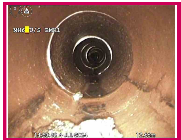
4, 00:01:23, 12.66 m Settled deposits, fine, 10% cross-sectional area loss
