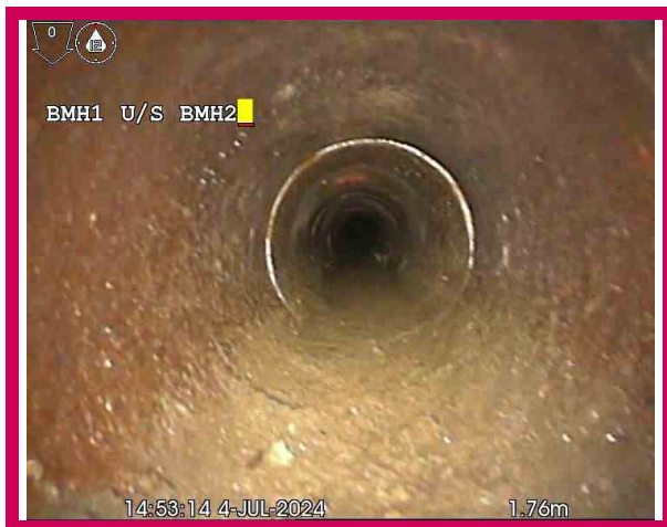
3, 00:00:15, 1.76 m Finish node, other special chamber, reference: UMRWP1, Line reduces to UMRWP1, not BMH2 as stated on screen.
