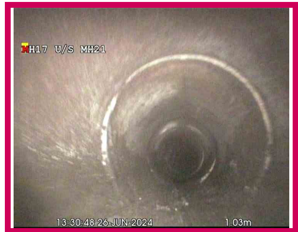
2, 00:00:09, 0.18 m Settled deposits, fine, 10% cross-sectional area loss, start
