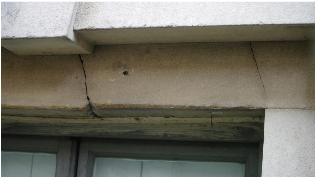
Figure 7 - Failed Lintel, offset crack. Additional flexural crack at bearing.
