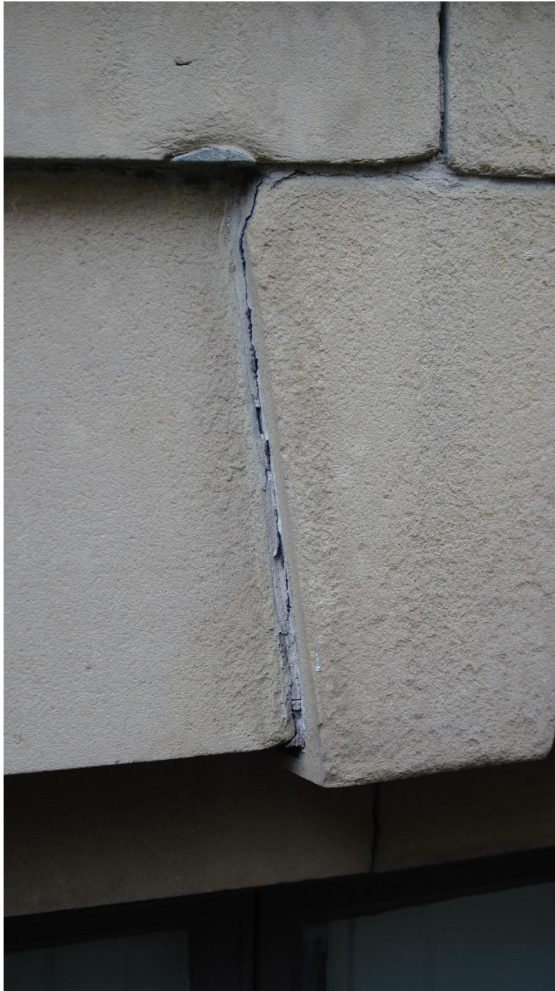
Figure 3 - Joint slippage around the keystone
