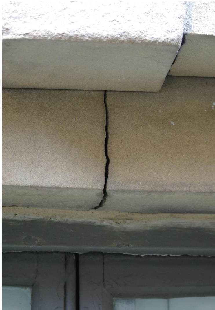
Figure 2 - Failed, cracked lintel – likely supported by the window frame
