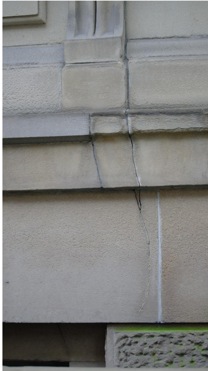
Figure 8 - Shear crack at bearing of voussoir of keystone lintel.
