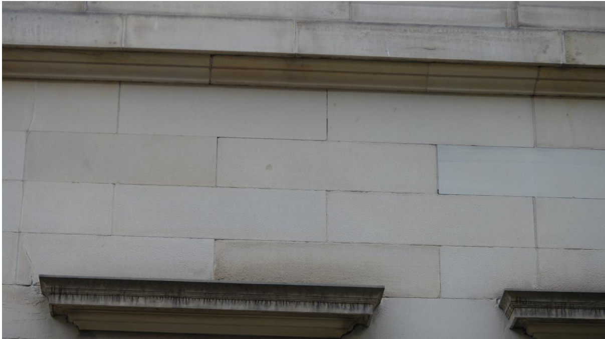
Figure 5 - Bed joint cracking over the window above, where the masonry has settled.
