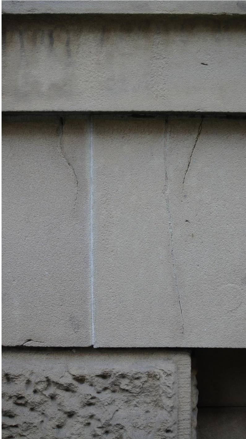
Figure 4 - Shear crack at left hand bearing of lintel, previously infilled with mortar
