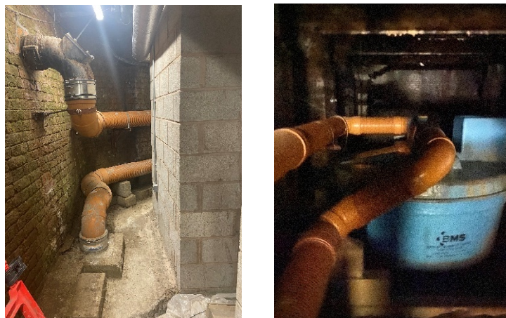
Figure 3—4 Surface water downpipe connecting Upper Yard to Lower Yard
