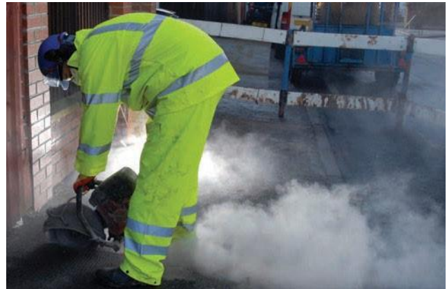
Figure 1 Construction dust levels during cutting and grinding / high dust levels
