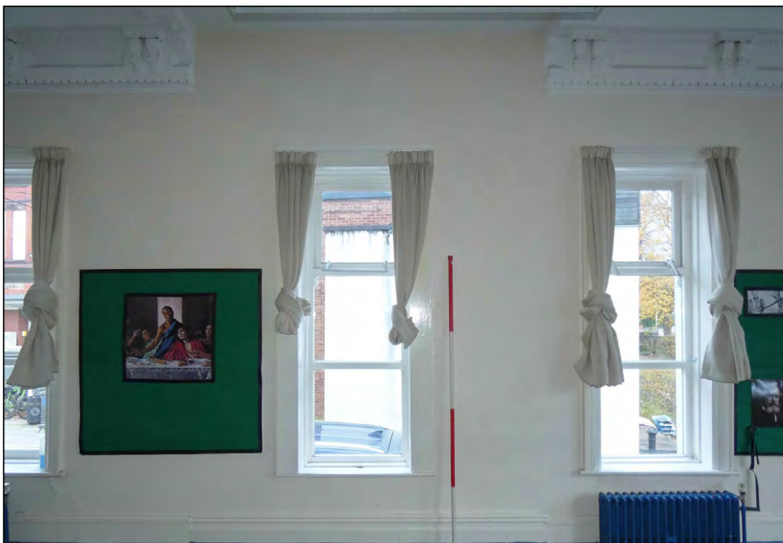
Appendix 2.50: Detail showing missing coving suggesting removal of fireplace from east wall of G10 (DI50) (Scale 2m)
