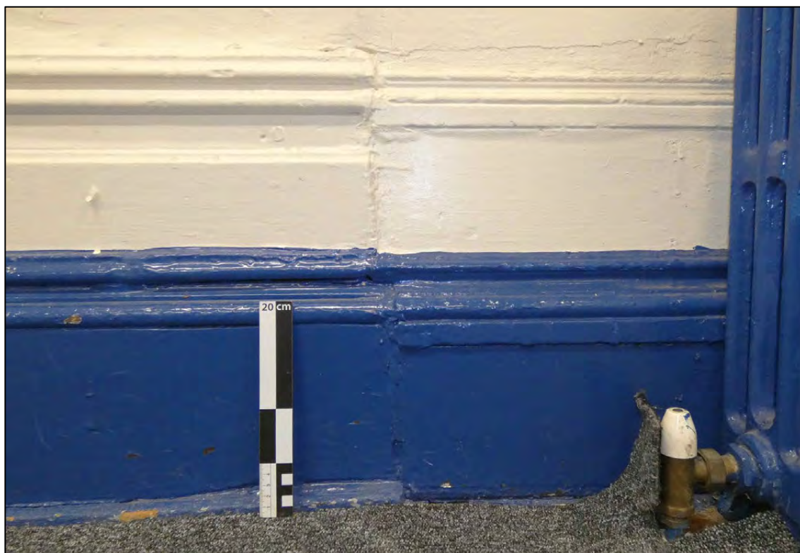
Appendix 2.51: Detail of skirting board misalignment east wall of G10 (D151) (Scale 20cm)
