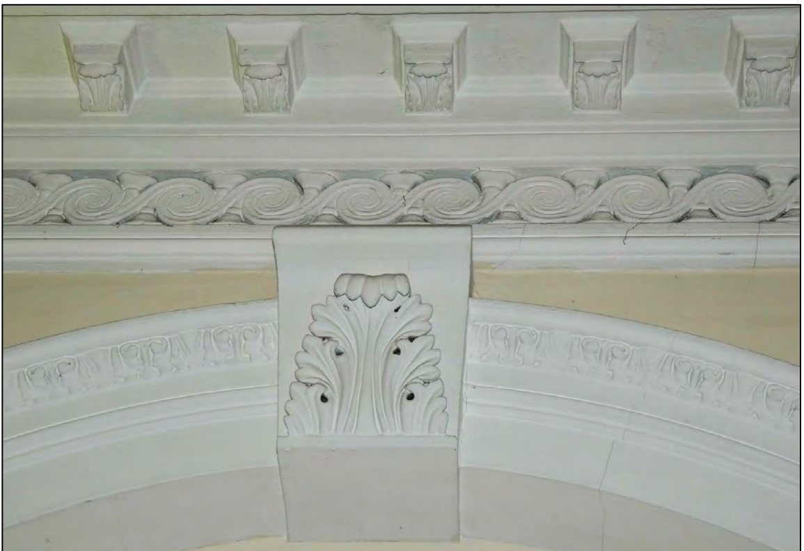
Appendix 2.38: Detail of keystone in archway south wall G4 (DI34)
