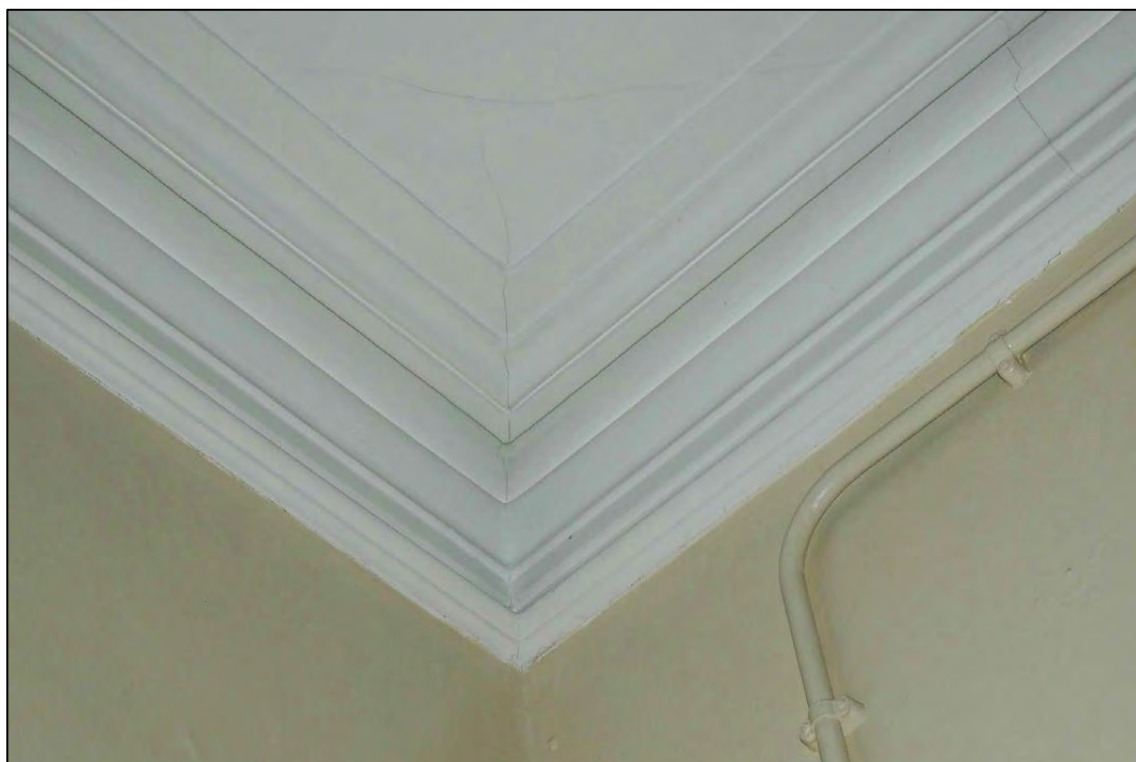
Appendix 2.121: Detail of coving in south-east corner F2 (D96)
