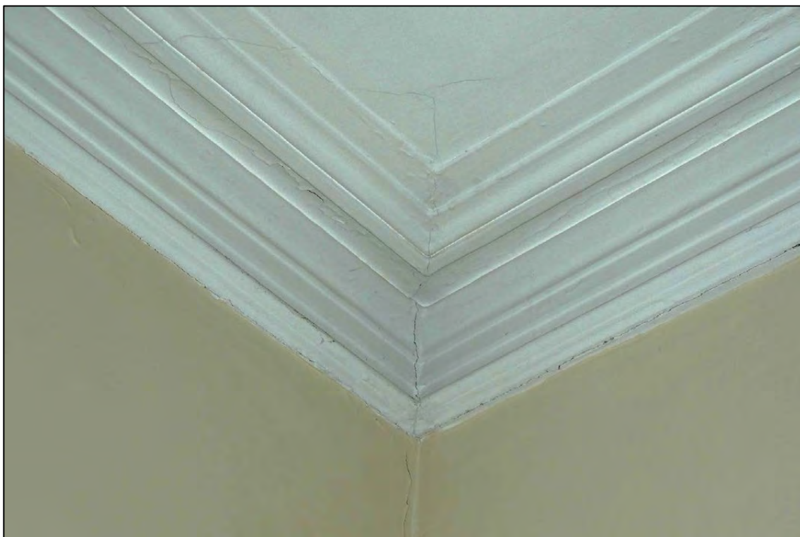
Appendix 2.97: Detail of coving in south-east corner F7 (D55)
