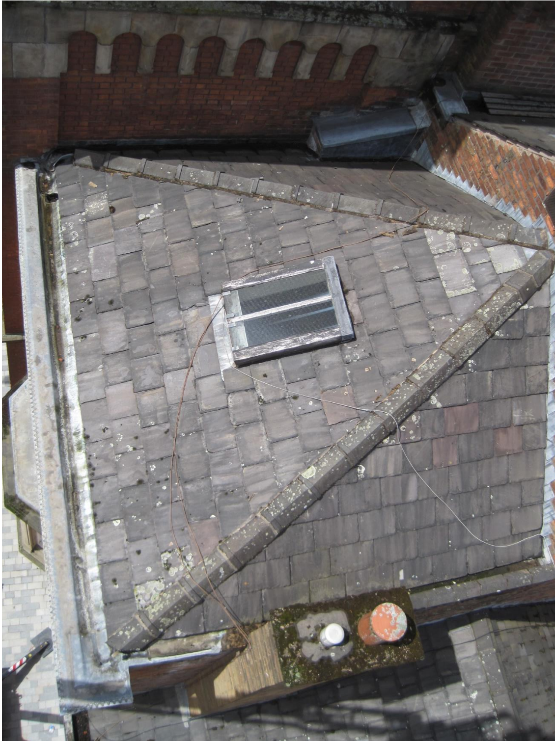
Fig 2: The west end roof of the Presbytery. The lead-lined gutter (left) is drained internally and is inaccessible for maintenance
