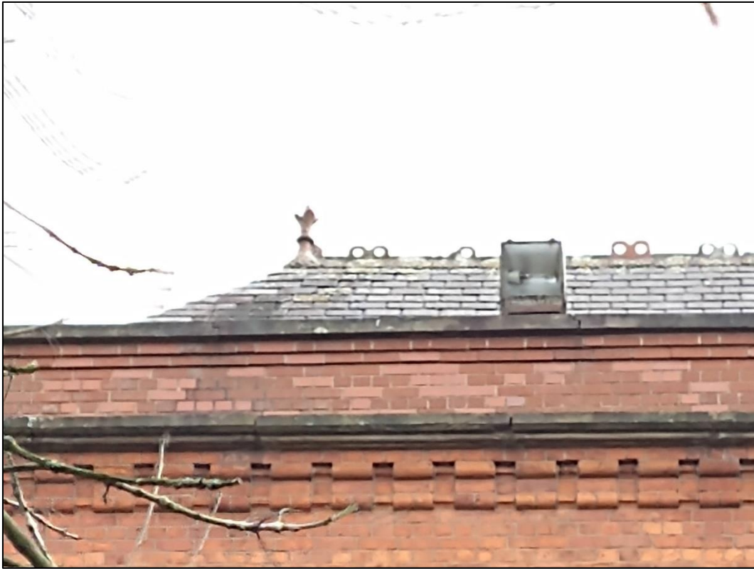
Plate 20: Example of security floodlight, located on the roof parapet.
