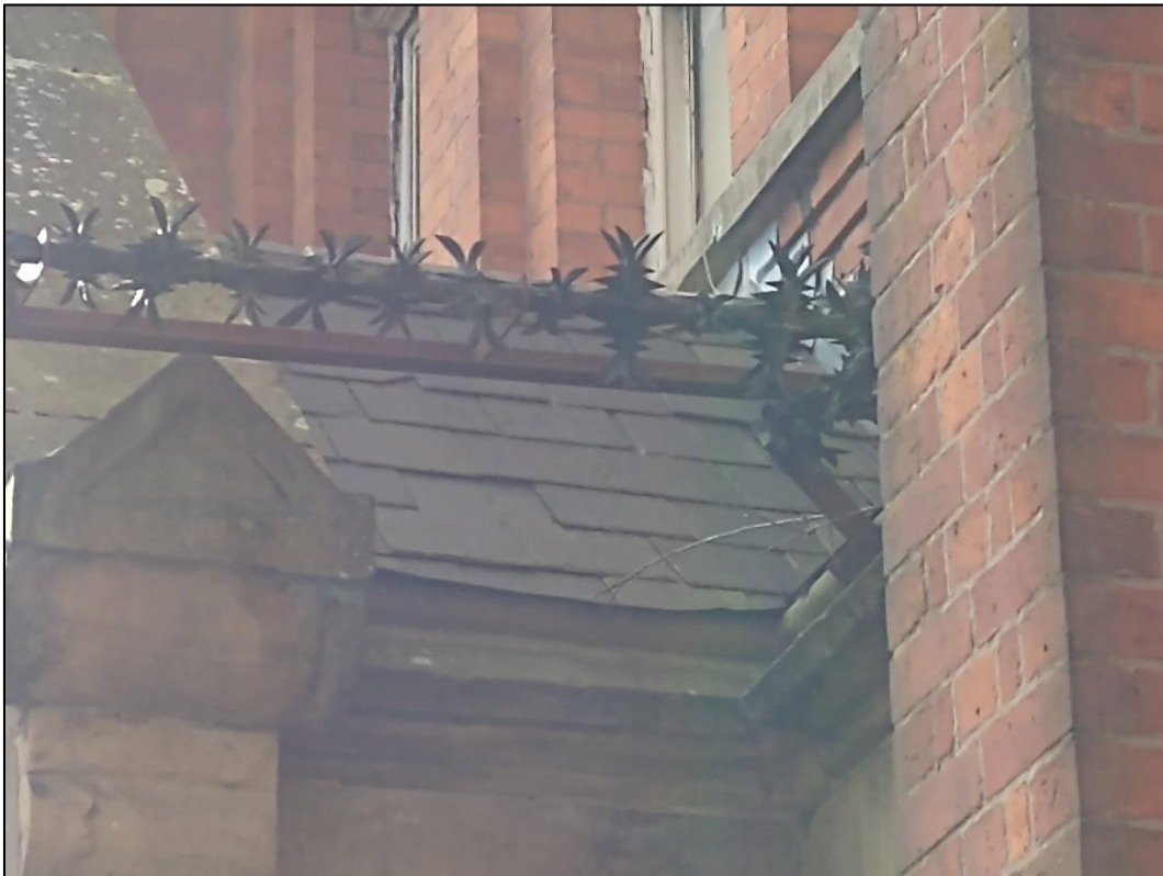
Plate 11: Gaps beneath slate tiles, present on the eastern porch of the building.
