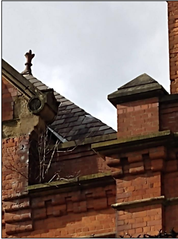
Plate 12: Lifted slate tiles on a hip, forming the section of roof above the clock tower. Small gaps in the lower stonework layer are also visible.
