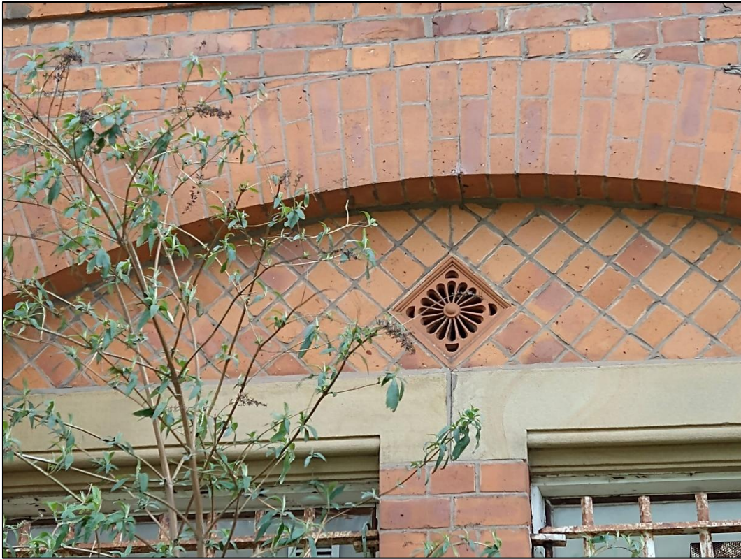
Plate 8: Example of decorative air vent, which were located throughout the building on multiple levels. Gaps in the vent cover were large enough for entry by bats, and a sizeable cavity was present behind each vent.
