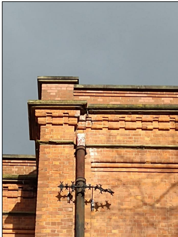
Plate 7: Example of gap in stonework above drainpipe, located on the southern façade.
