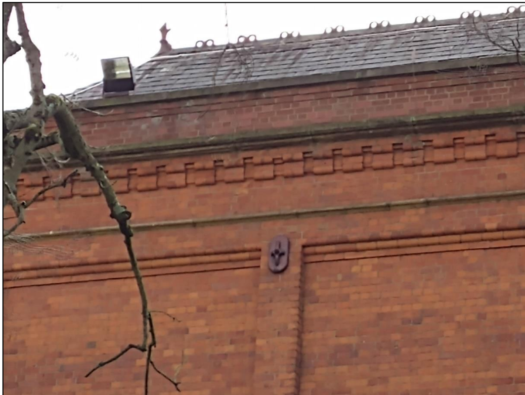
Plate 13: Zoomed view of slate roof showing small gaps beneath slate tiles and beneath ridge tiles.
