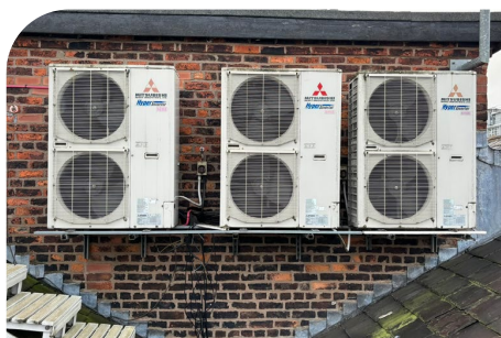
Fig 4. Existing VRF outdoor units
