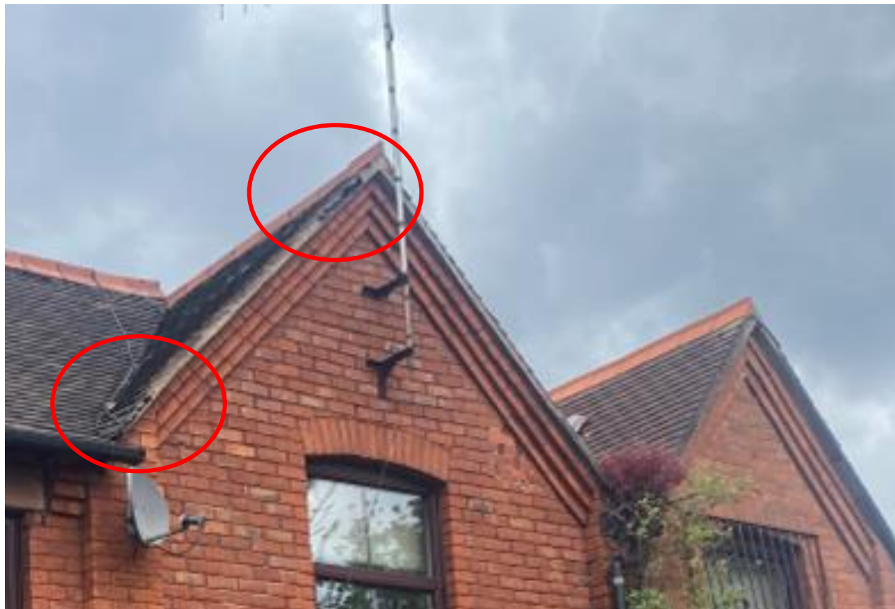
Photo 4: Close up of missing mortar present on southern elevation of B1.
