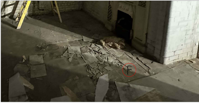
BASEMENT FLOORING - POOR CONDITION
