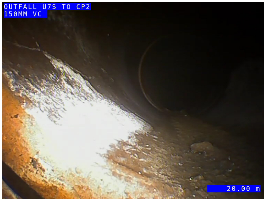
Photo: 3_3_19_A.jpg 20m, Joint displaced, medium
