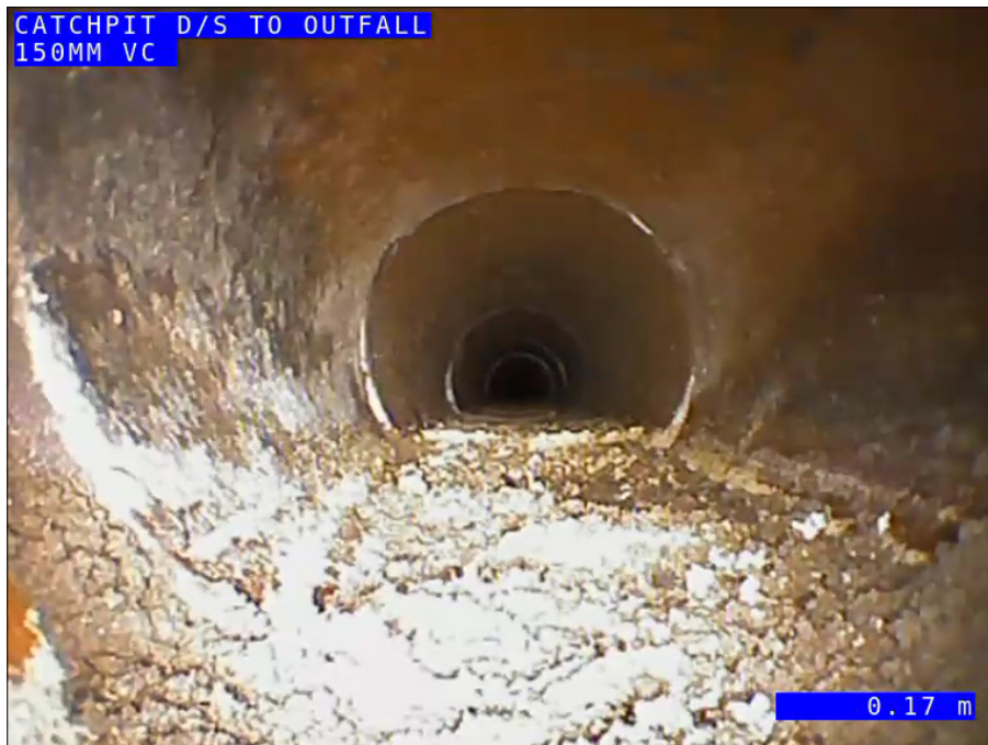
Photo: 1_1_8_A.jpg 0.08m, Settled deposits, fine, 10% cross-sectional area loss, Start
