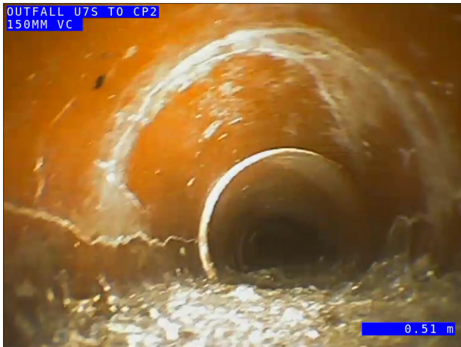
Photo: 3_3_14_A.jpg 0.51m, Settled deposits, fine, 10% cross-sectional area loss
