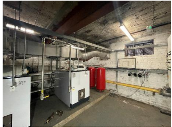
Figure 96: The basement boiler room (looking east)
