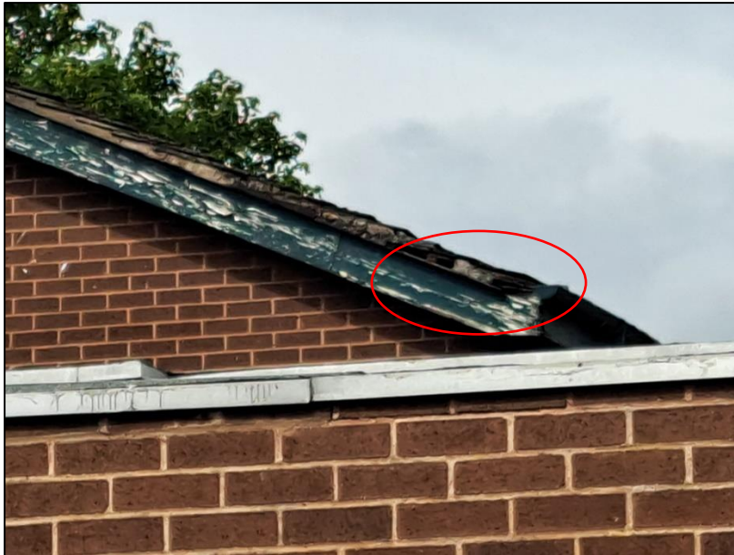
Photograph 2 showing a gap on the verge at the southeast gable
