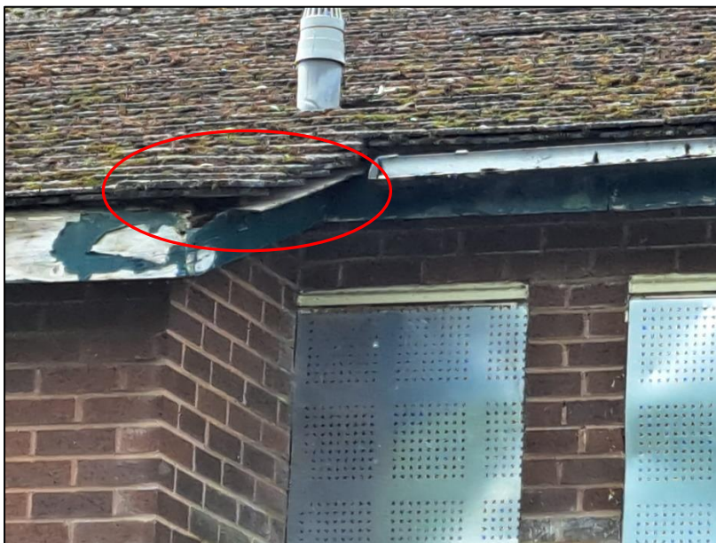
Photograph 3 showing a gap at the northeast edge of the main roof
