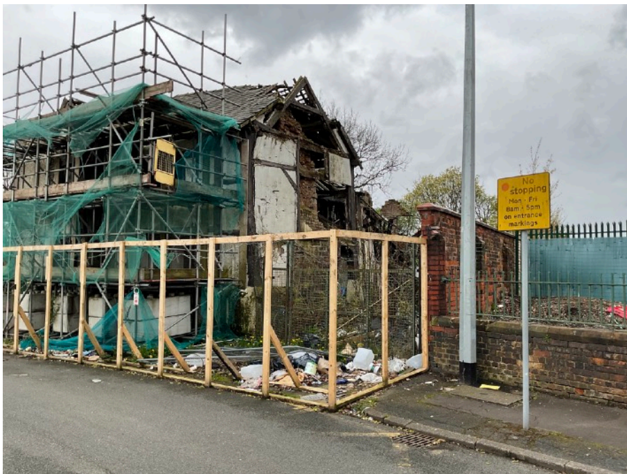
North gable. Panels are detaching.
