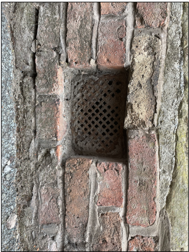
1) Cast Iron vent
