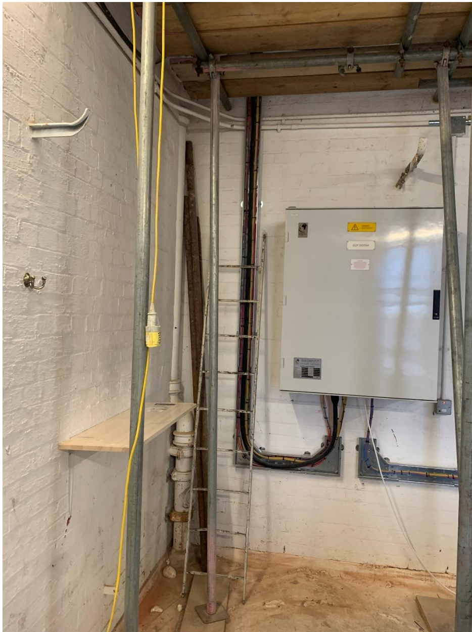
Figure 6 – Example of a TR cabinet for a similar structure – also located in a back-of-house/plant room area.
