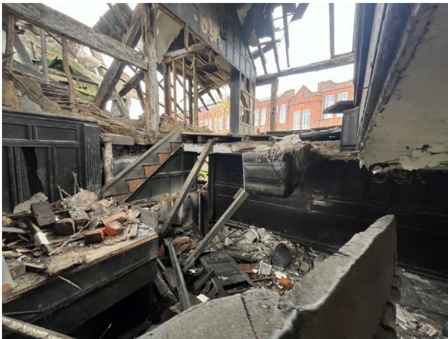
Much of the framing has been lost in the main body of the house.
