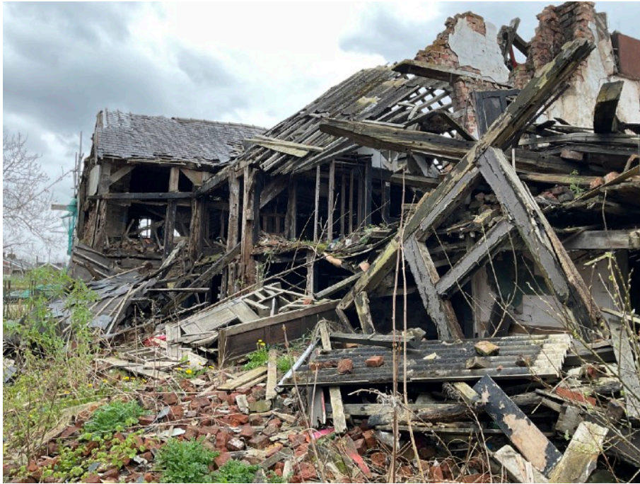
The rear is in a state of collapse.
