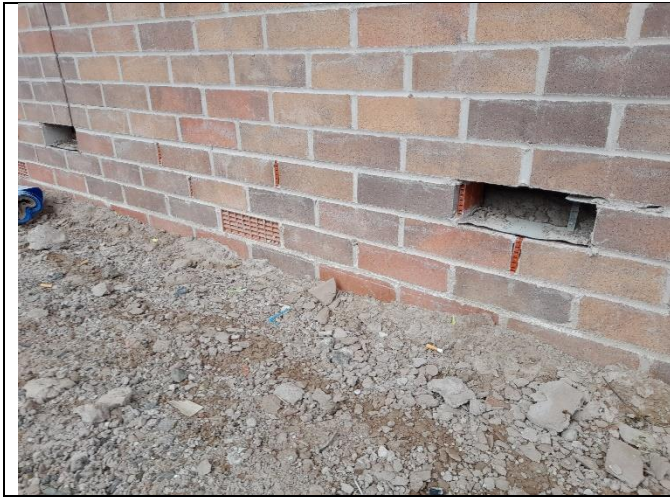
Evidence of airbricks.
