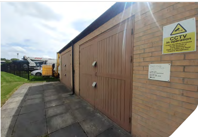
Photo 08: Electricity substation on site
