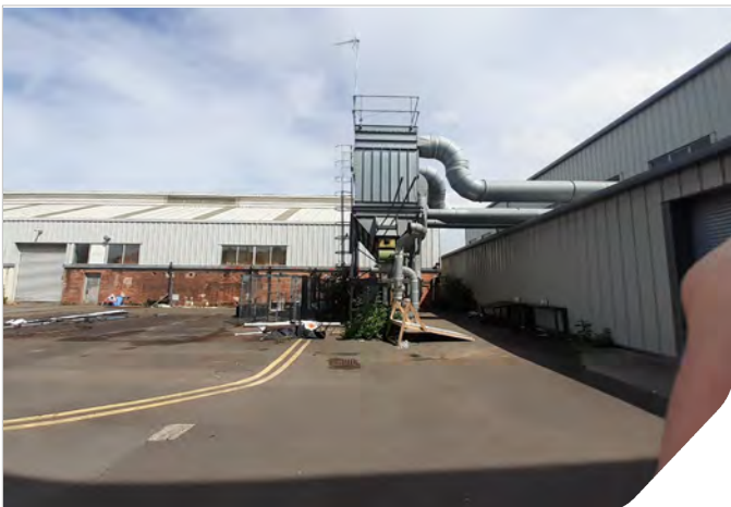
Photo 01: Ventilation or fume extraction system in central yard
