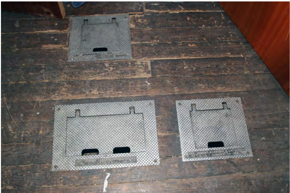
Plate 13. Stage, west side, electrical sockets in floor, viewed from east.
