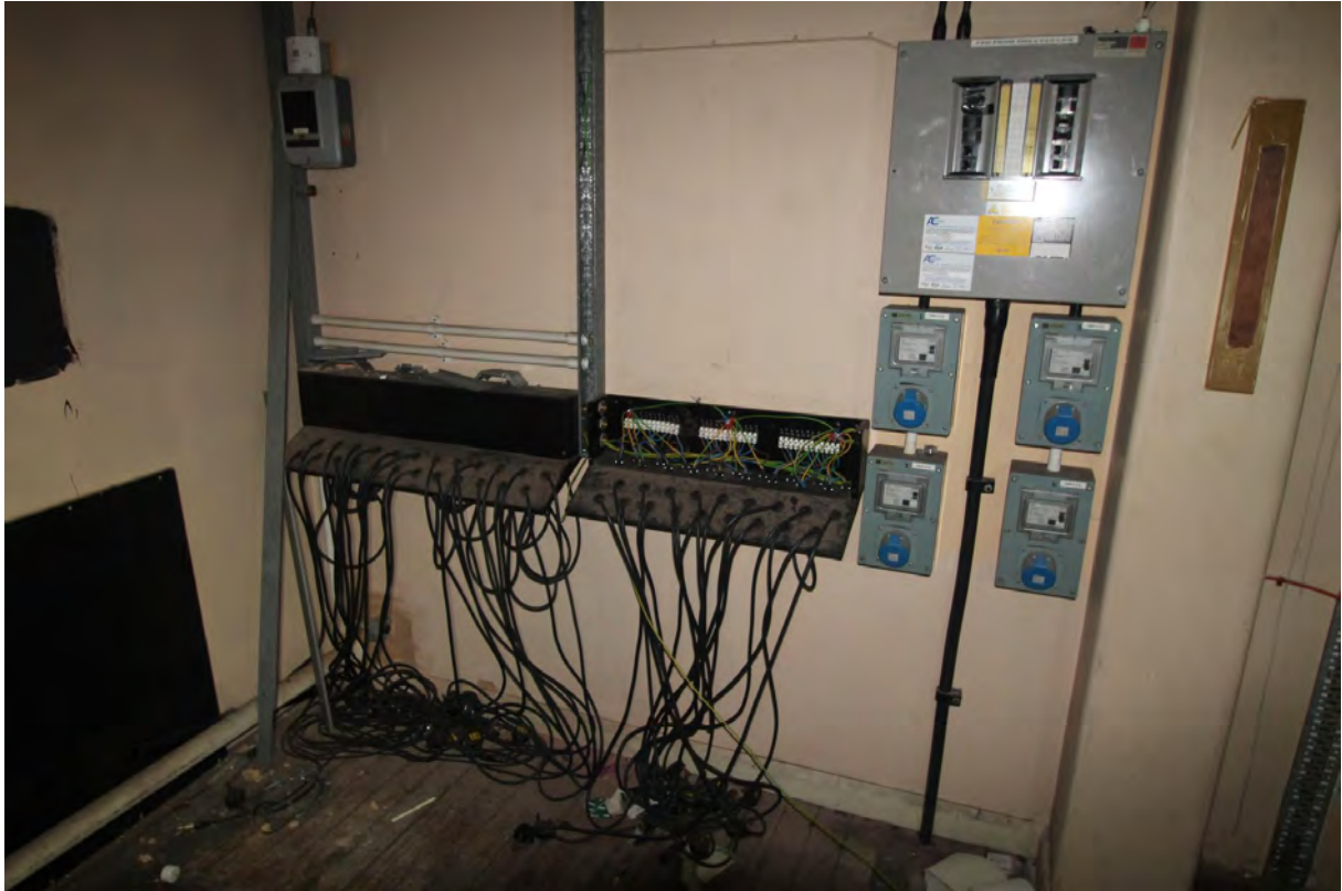
Plate 14. Stage, east side, electrical controls, viewed from north.
