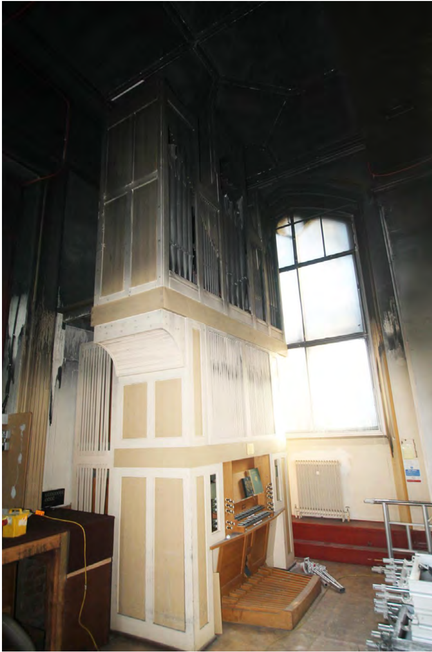
Plate 1. Fire damaged organ, viewed from west.
