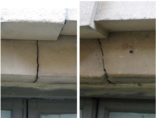
Figure 26 Photographs showing failed lintels to WIN-004 on George Street (left) and WIN-010 on Princess Street (right)
