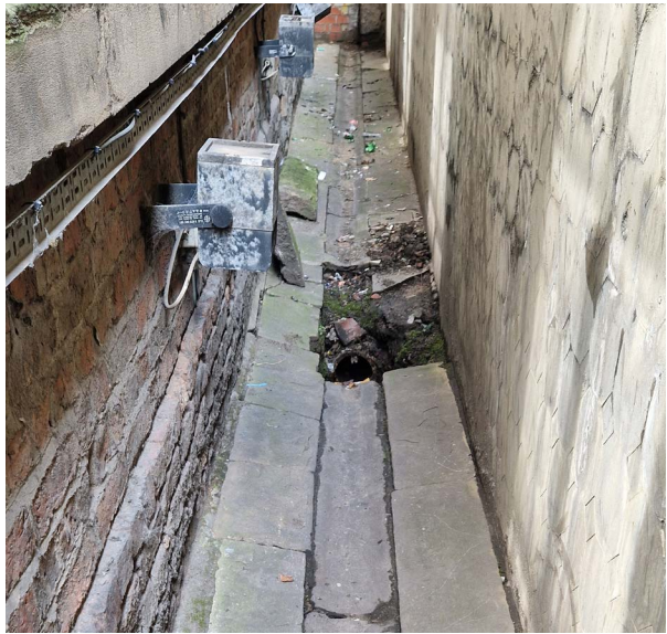
Figure 23 Photograph showing cracked paving slabs and broken out gully
