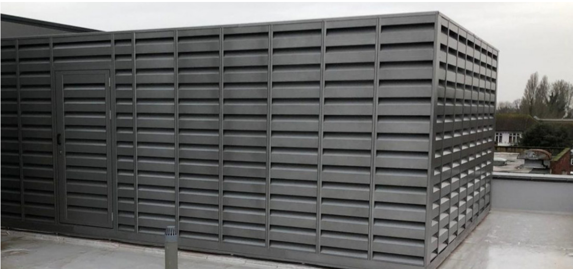
Accoustic Louvred Plant Panel
