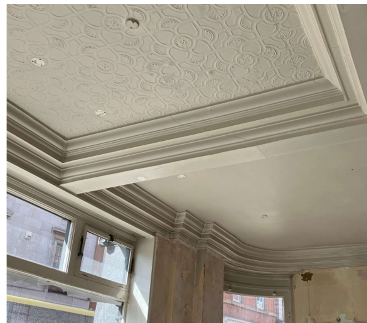
Figure 16 – Superficial Cracking Witnessed to Existing Ceiling / Coving
