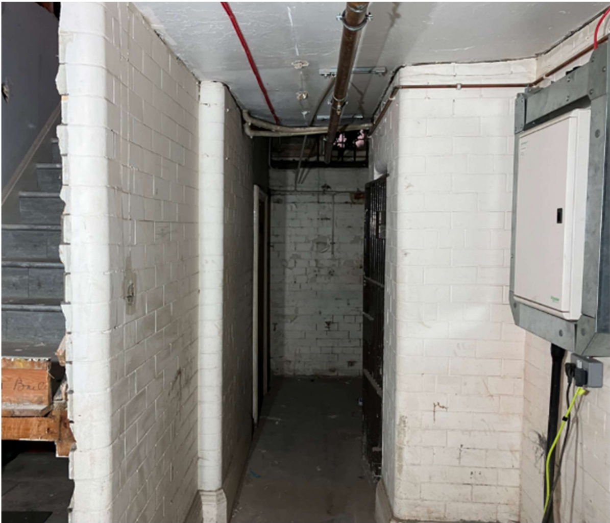
Figure 5 – View in Existing Basement (Electrical Distribution Board and Ceiling Level Services Visible)
