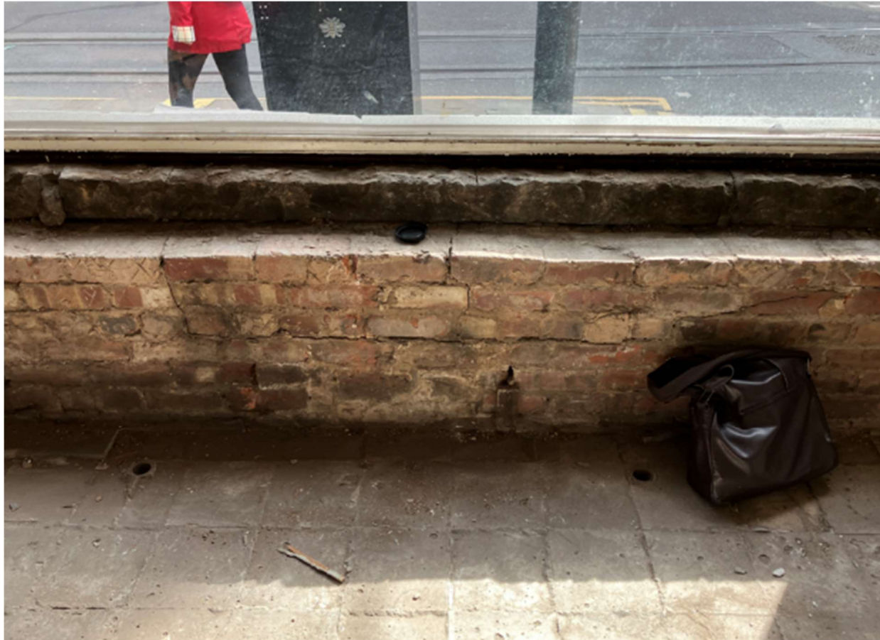
Figure 17 – Loose Masonry / Cracking to Brickwork Cills to Cross Street Elevation
