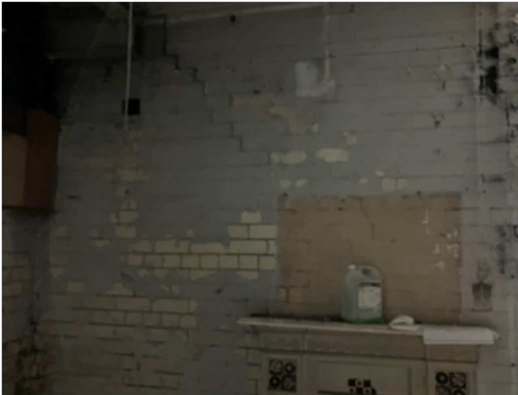
Figure 8 – Masonry Cracking to Existing Chimney Structure
