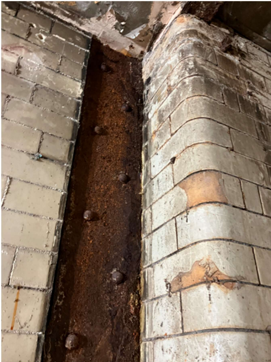
Figure 7 – Embedded Steel Column Showing Signs of Rusting
