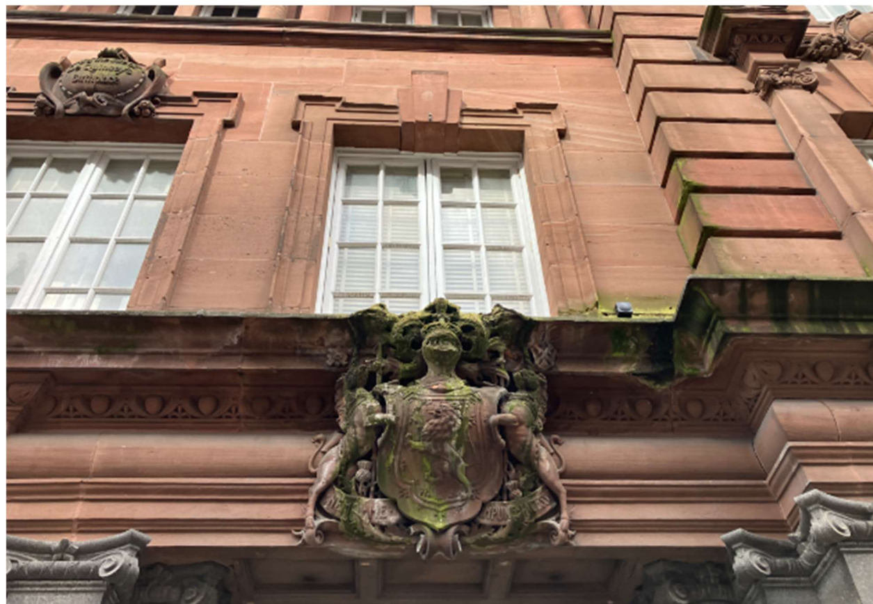
Figure 23 – Minor Moss Staining to Stonework
