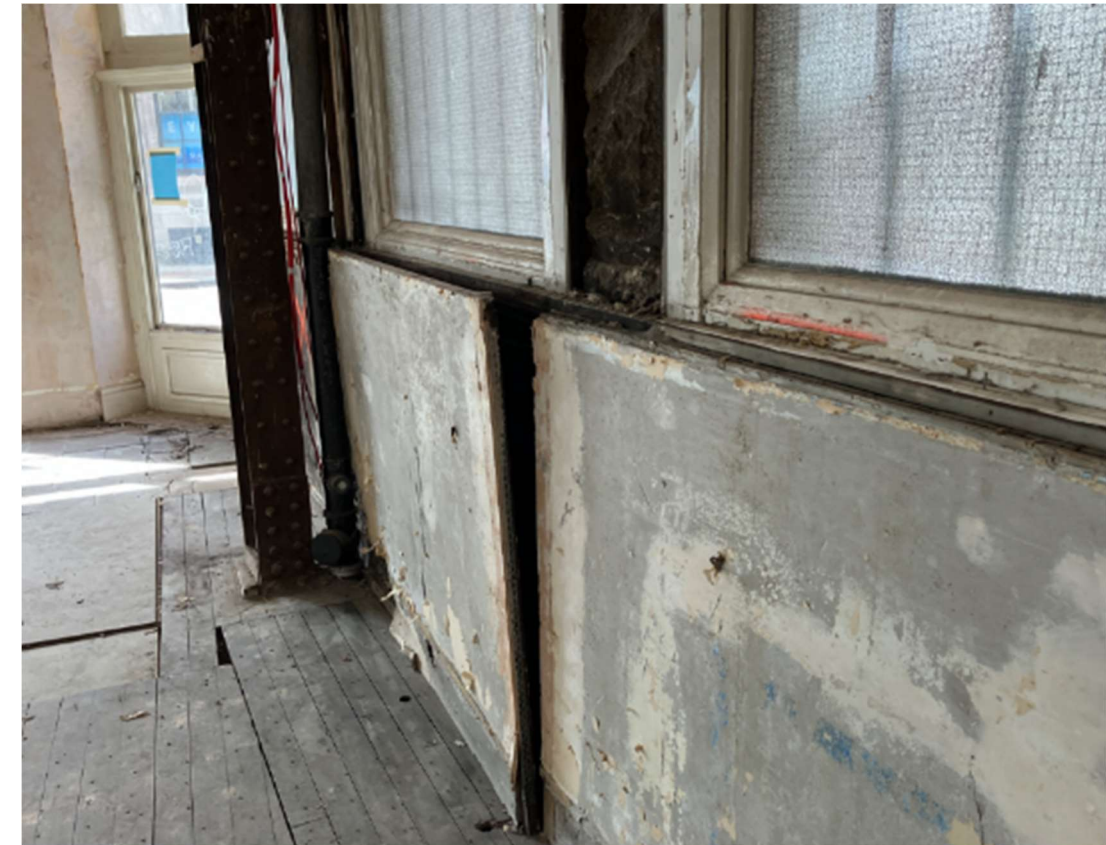
Figure 18 – Loose Plasterboard Panelling to Rear Elevation
