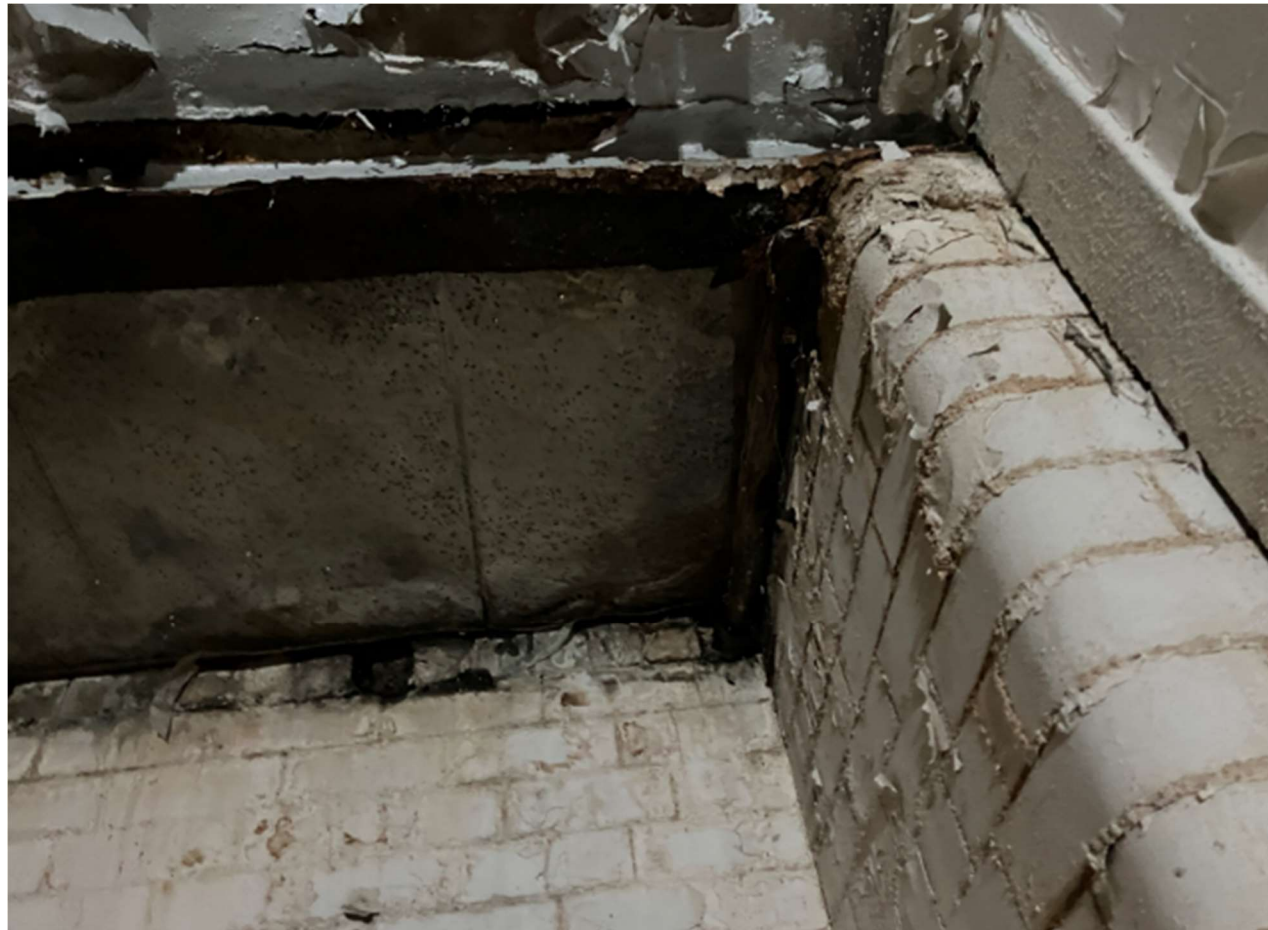
Figure 13 – View on Former Pavement Smoke Vent Showing Slab Infill and Corroded Steel Support Member
