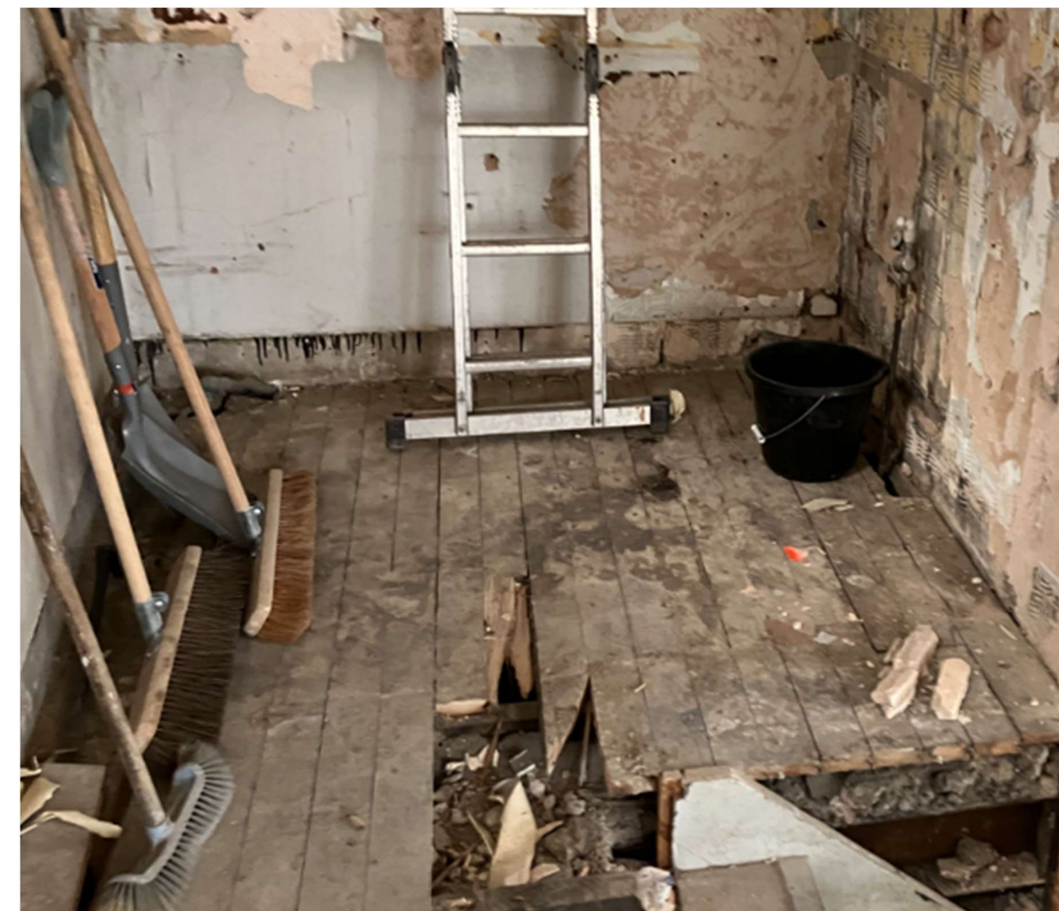
Figure 20 – Damaged Floor Board Finishes to Top of Basement Access Stair
