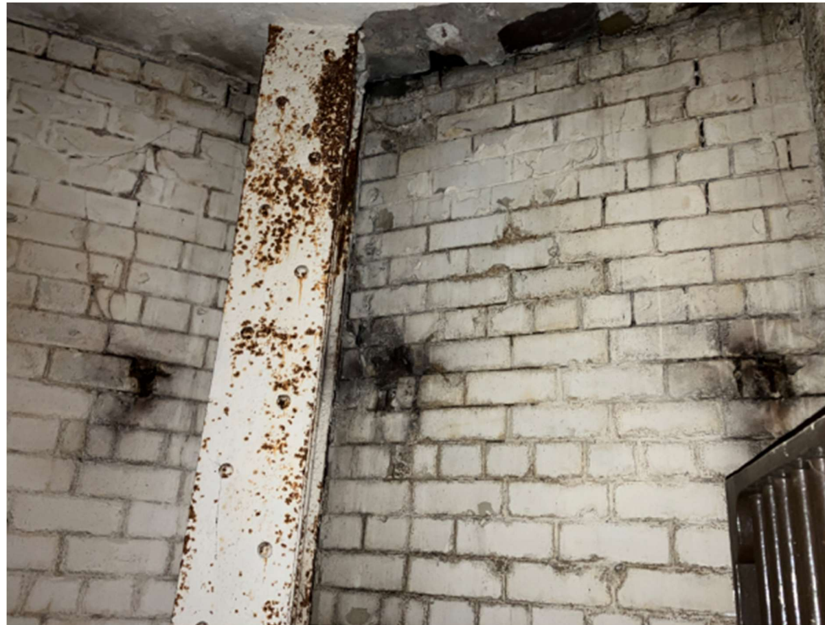
Figure 9 – Steel Support Column Showing Signs of Surface Rusting
