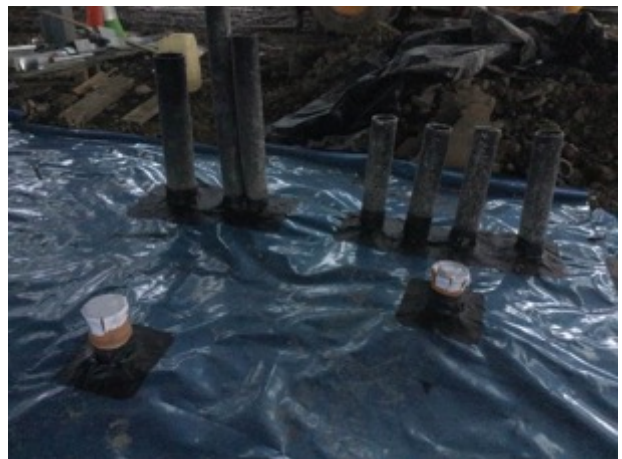
Pipe penetration details sealed with SAGM within Unit B office area.
