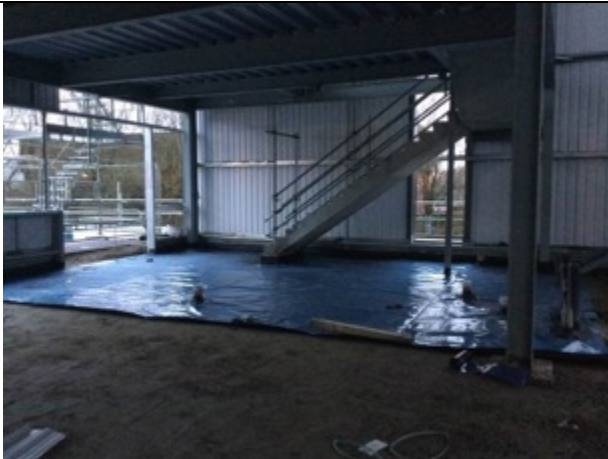
Overview to Unit D membrane line out.
