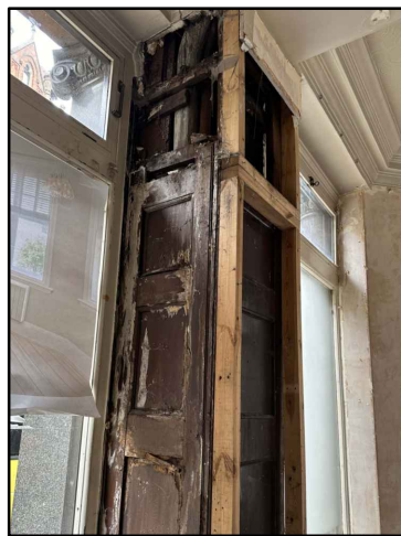
GROUND FLOOR HEAVY WATER DAMAGE TO PANELED CASINGS
