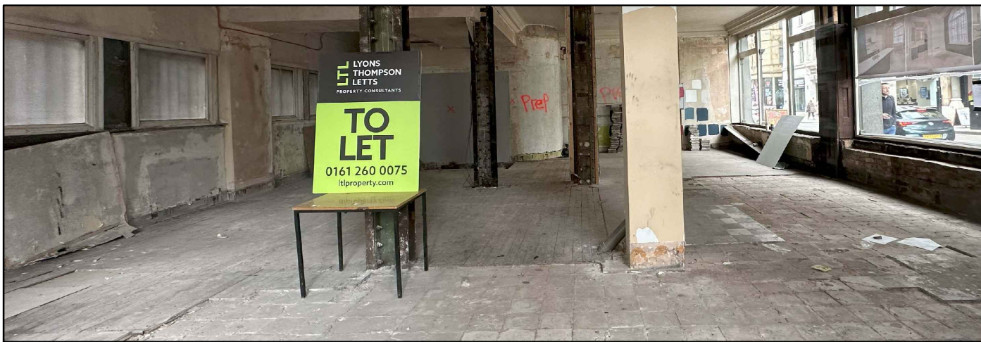
GROUND FLOOR NO SKIRTINGS THROUGHOUT SITE
