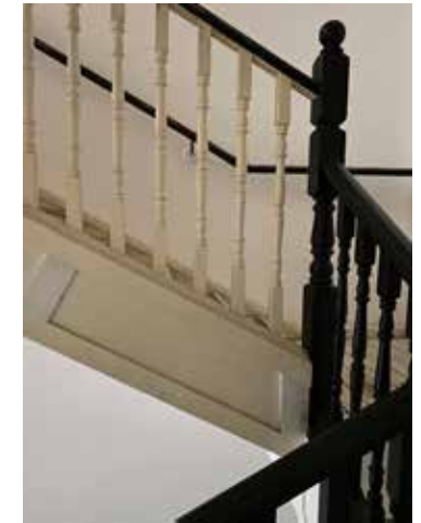
Plate 3.4.164 change in paint colour halfway up the flight from ground to first, also note poor quality paneling
