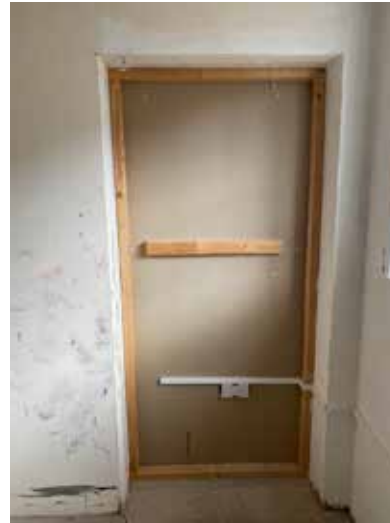
Plate 3.4.144 S.02 blocked opening to S.01
