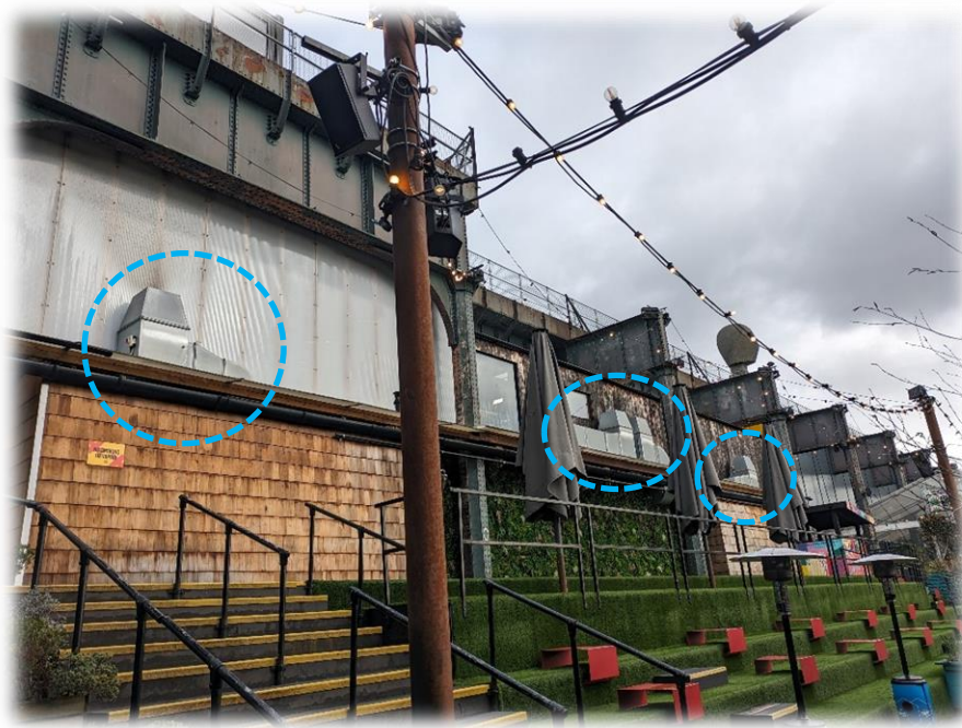
Figure 7 – ‘Freight Island’ dedicated commercial grade kitchen extraction systems – Typical 4no extraction systems via the rear façade to Mayfield Park.
