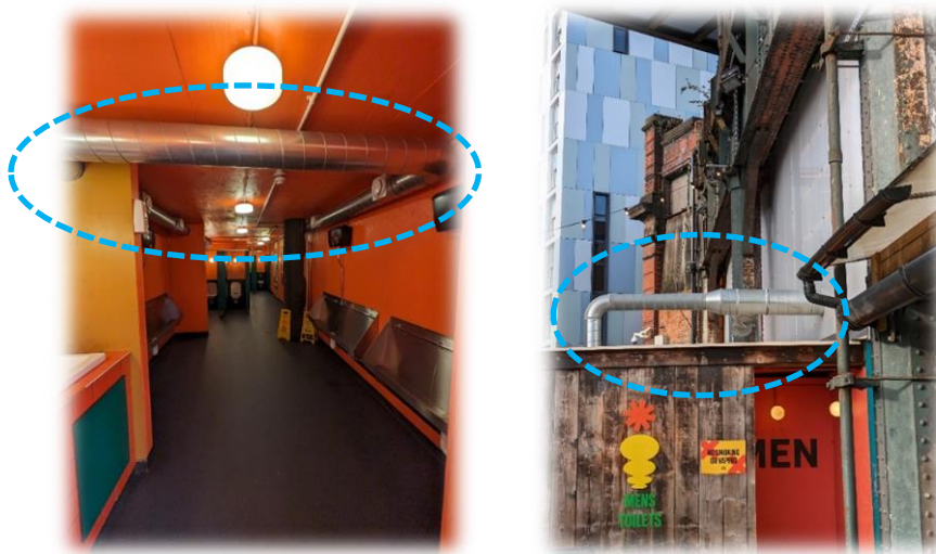
Figure 8 & 9 – Freight Island WC ventilation system via dedicated ducted central extract system.
