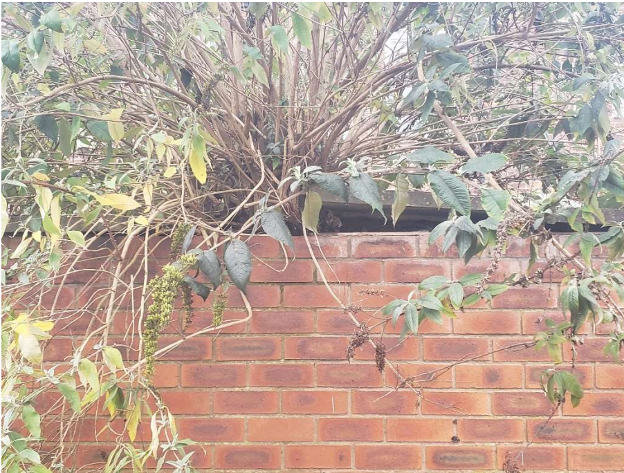
Figure B.9 Gap at top of wall on northern boundary which provides ingress into wall cavity
