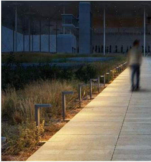
Figure 19: low level bollards to illuminate the walkway
