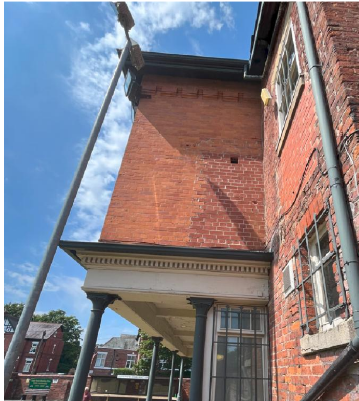
Image 5 – August 2024 photograph showing former external first floor door opening which is clearly identifiable as a different brick type has been used.
