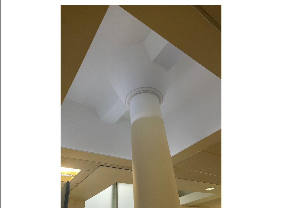
Figure 12: A typical example of the deep, dropped ceilings across the unit, which obscure or conceal the original column capitals.
