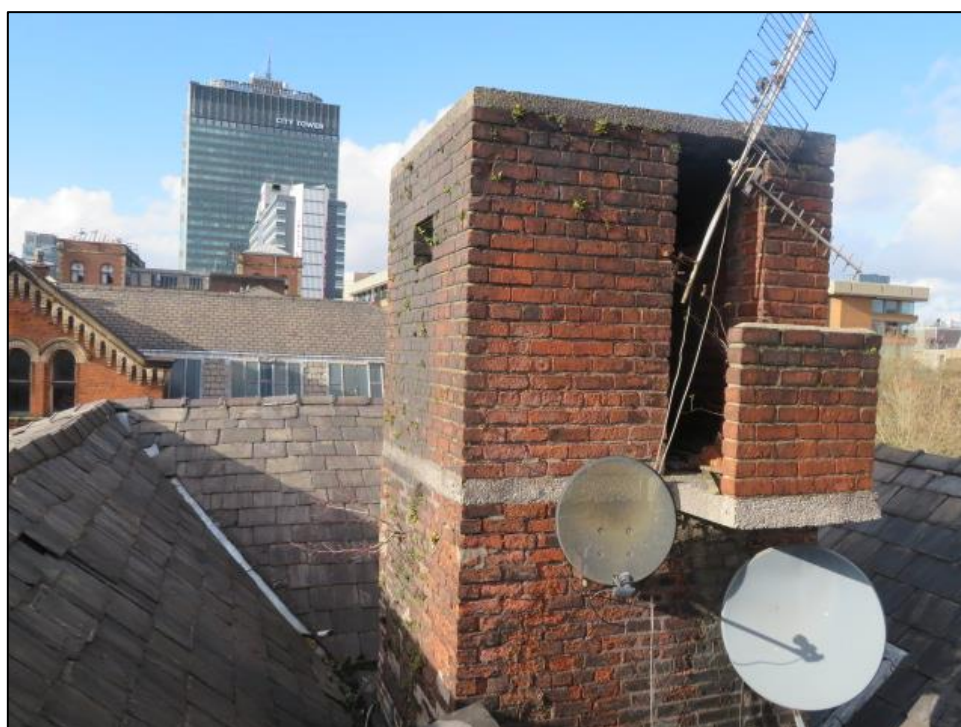
Figure 6: Photograph of brick shaft housing showing concrete slabs, spalling brick and vegetation growth.
