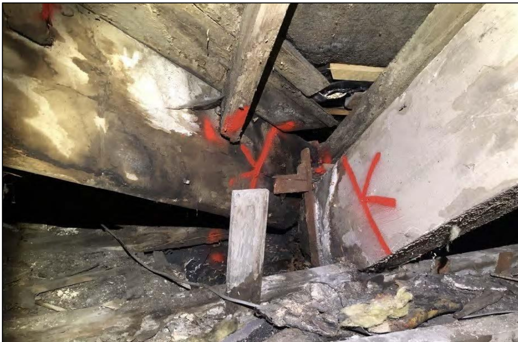
Figure 12: Photograph of roof structure showing water damage (June 2021).
