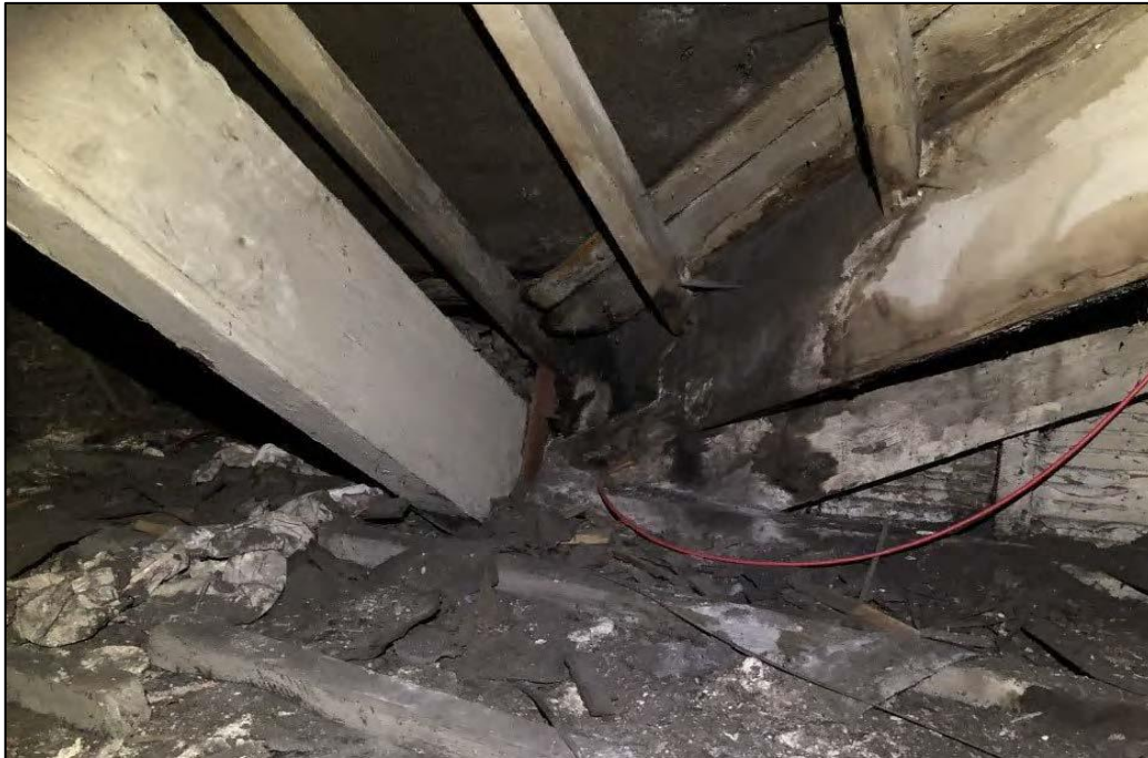
Figure 11: Photograph of roof structure showing water damage (June 2021).
