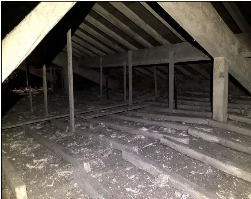
Figure 9: Photograph of roof structure showing extensive deposited 'torching' (June 2021).
