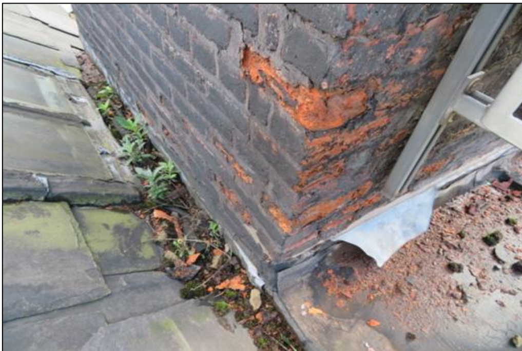
Figure 8: Photograph showing detail of brick shaft with roof valley. The design of which presents an inherent defect vulnerable to failure and build-up of vegetation.
