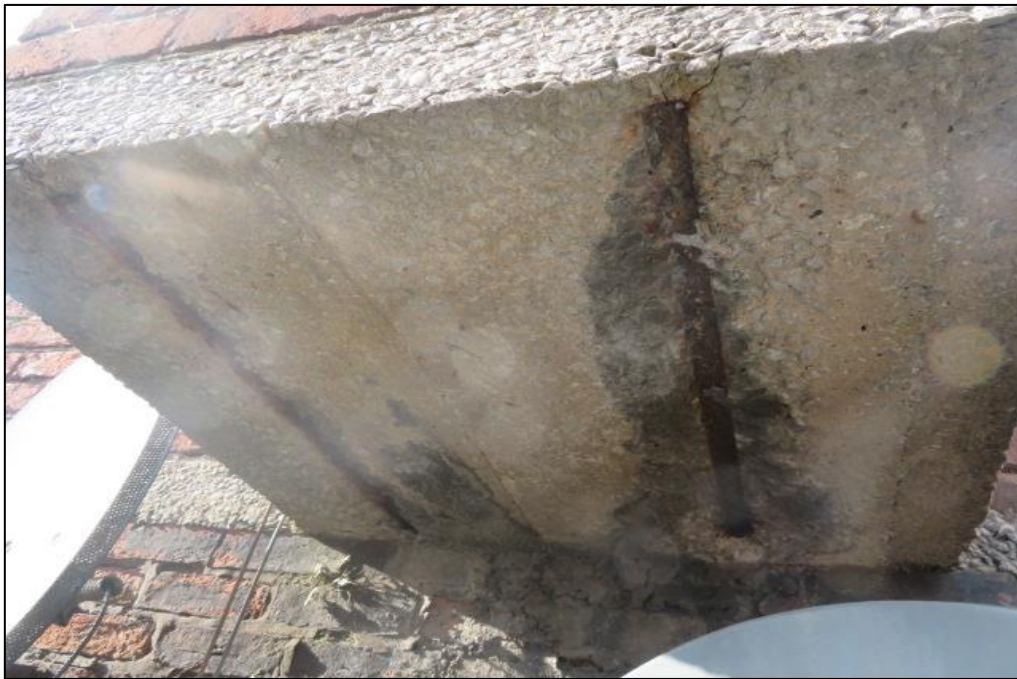
Figure 7: Photograph showing delaminated concrete and spalling brick of the hoist overrun.
