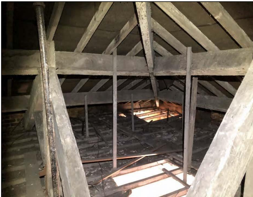
Figure 10: Photograph of roof structure showing extensive deposited 'torching' and failed areas of lath and plaster ceiling (June 2021).
