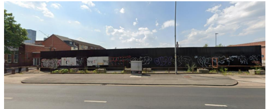
Photo 1 – New Fibre cabinet installed on Cheetham Hill Road
