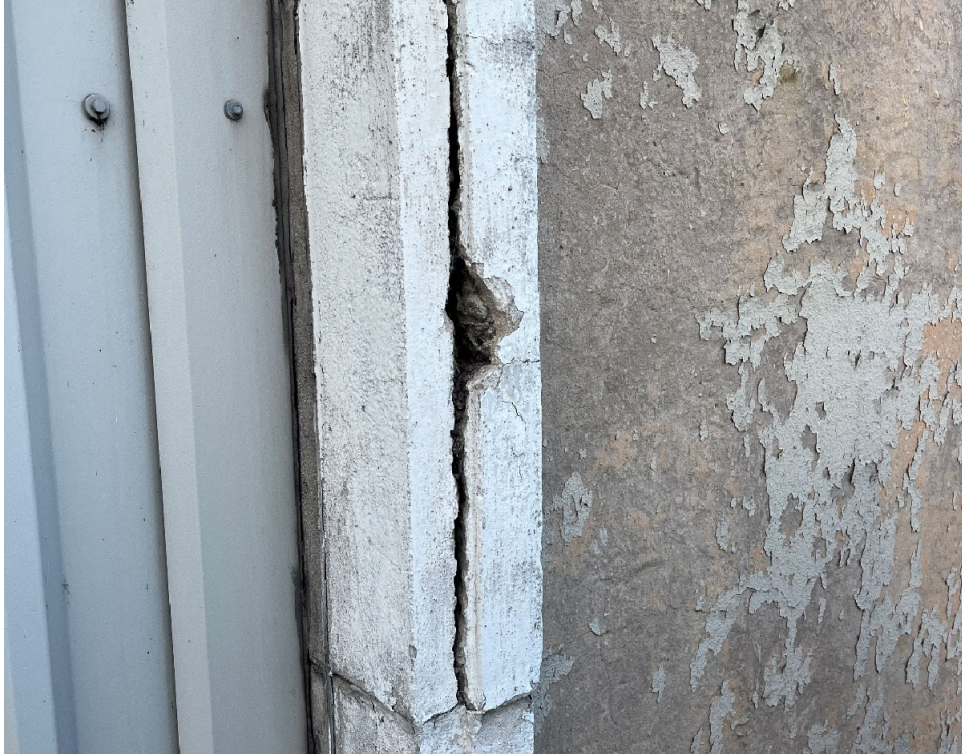
Photo 8. Spalling window jamb to right-hand side of window 8
