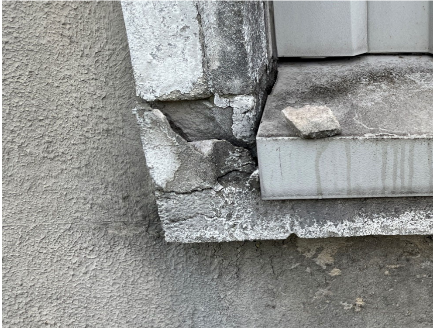
Photo 14. Spalling to bottom left-hand corner of window 6 surround
