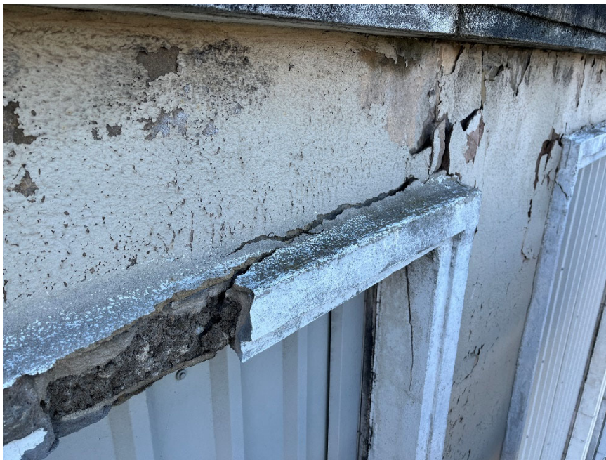
Photo 15. Large section fallen from the lintel of window 4
