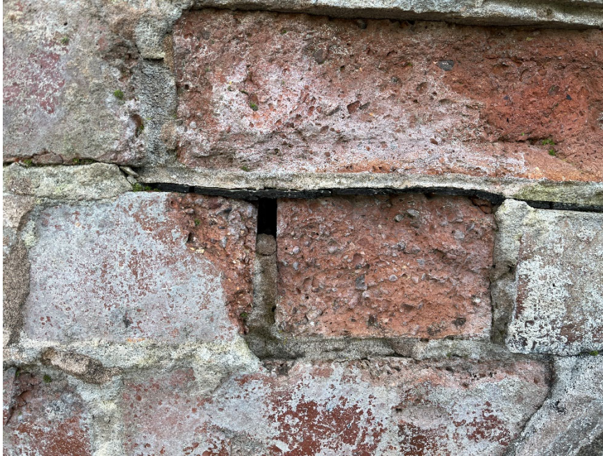
Photo 20. Decayed bitumen DPM to parapet wall
