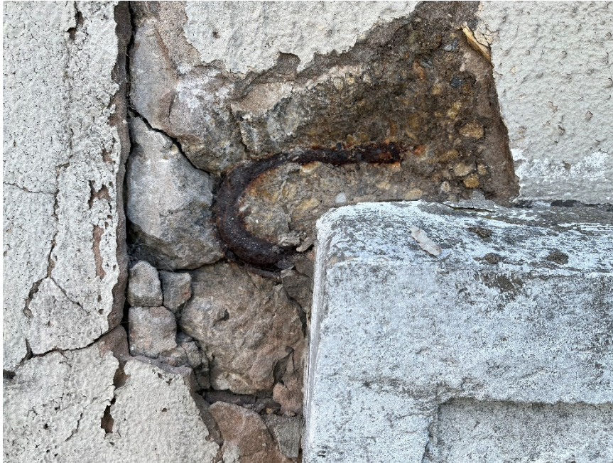
Photo 18. Exposed bottom reinforcing bar to left-hand side of window 1 lintel
