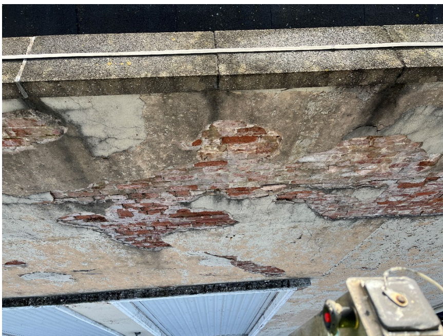
Photo 19. Delamination of render coating to parapet
