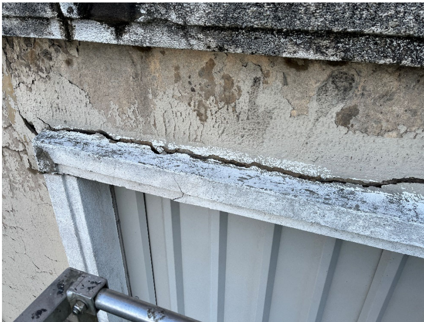
Photo 11. Cracking to left-hand side of window 7
