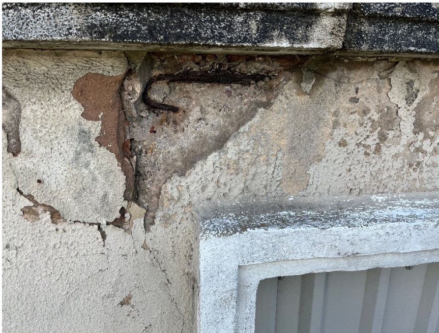
Photo 17. Hooked end of reinforcing bar visible to window 3 head
