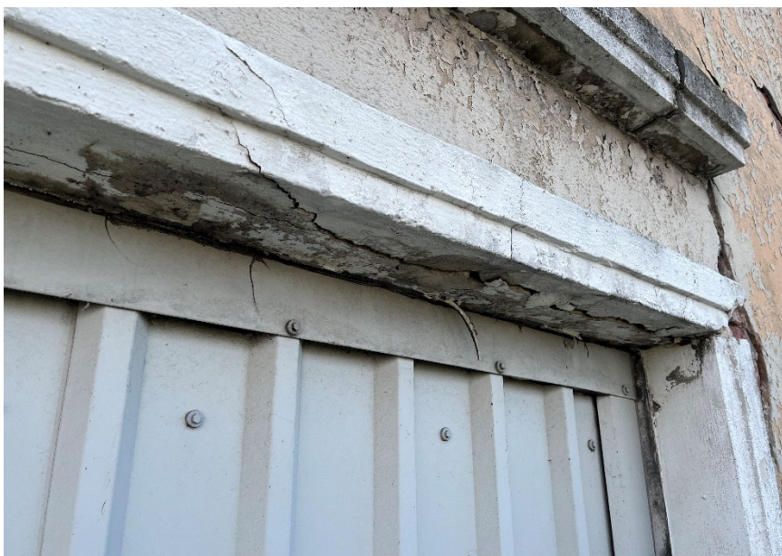
Photo 7. Longitudinal crack to soffit of concrete lintel
