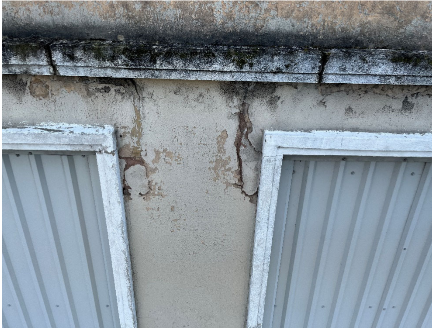
Photo 10. Cracking and spalling between windows 7 and 8
