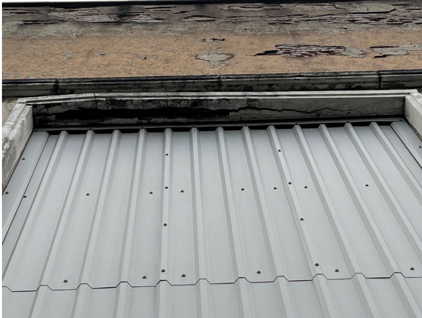
Photo 12. Head of window 6 with severe spalling and risk of debris falling
