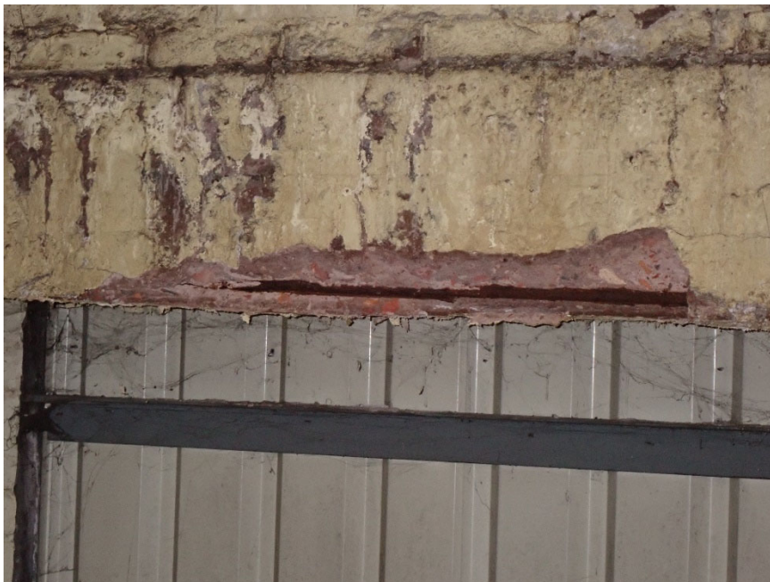
Photo 24. Spalling of internal face of window 8 internal lintel
