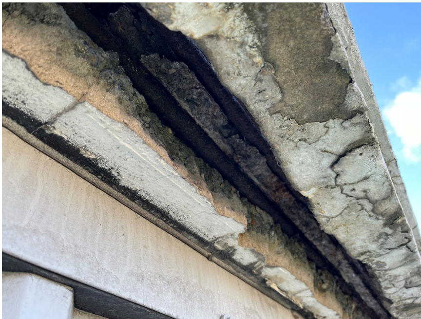
Photo 13. Reinforcing bars visible to underside of window 6 lintel
