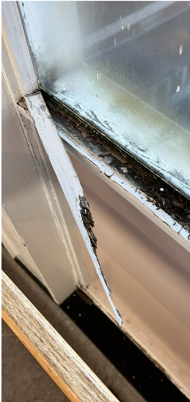
Figure7: Image displaying decayed elements in envelope
