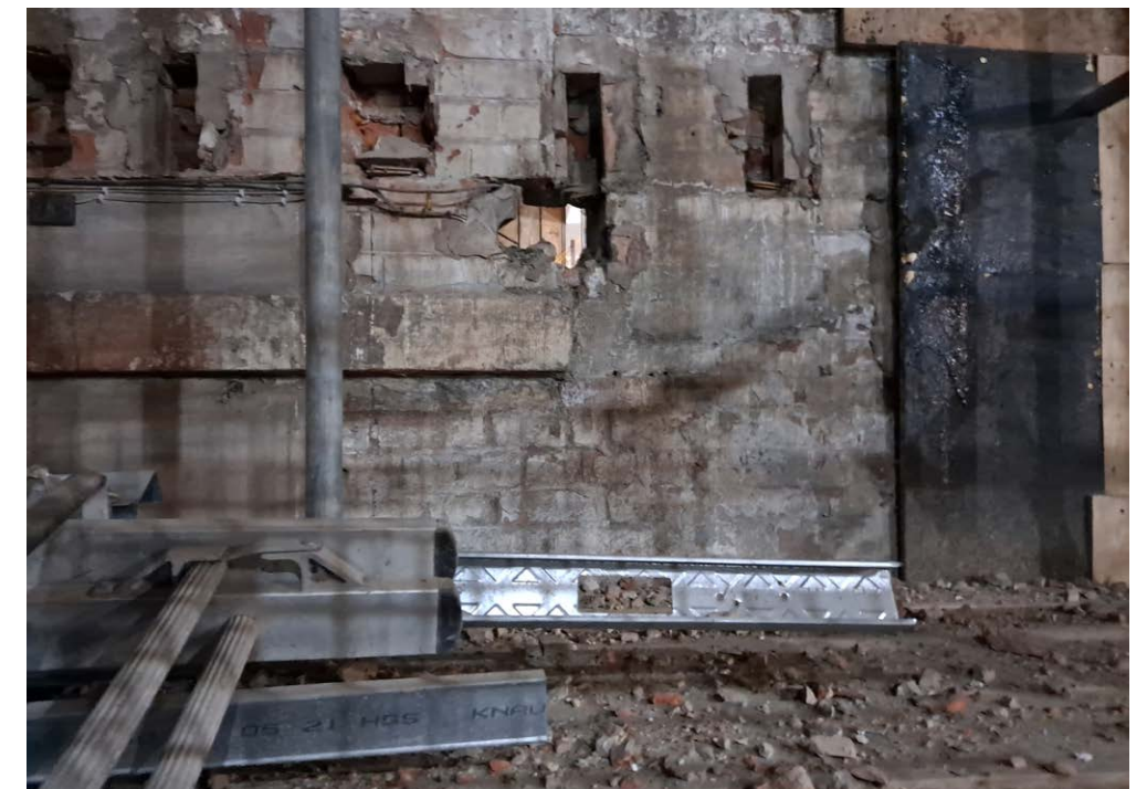
Image of the damaged internal brickwall proposed to be lined
