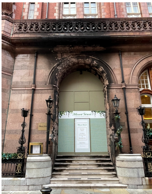
Photographs showing fire damage to Mount Street entrance.
