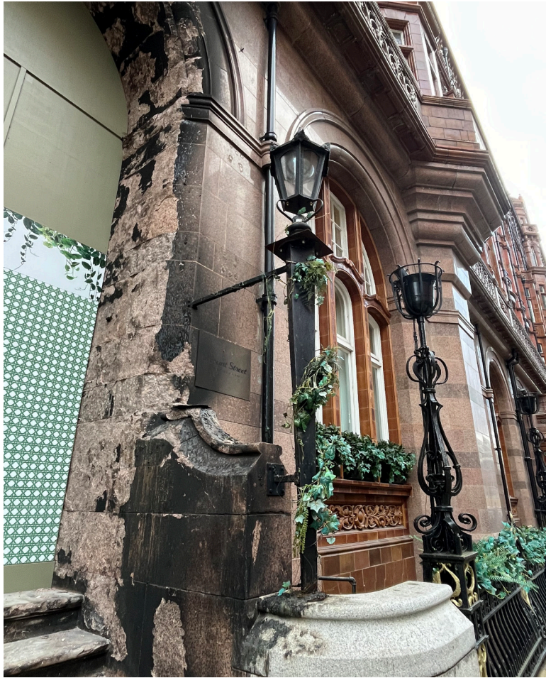
Photograph showing fire damage to right hand side of Mount Street entrance.
