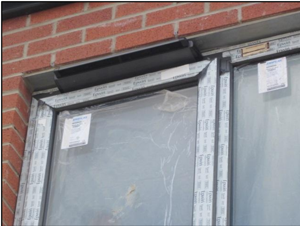
Photograph 8. Titan V75/C75 acoustic ventilator, plot 1 - front bedroom
