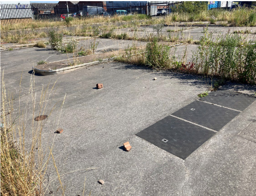
Refueling plinths & a Series of Manhole Covers
