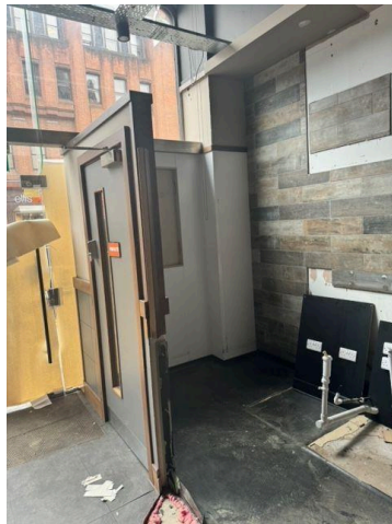
9 - free standing / non original door frame / partition to be removed
