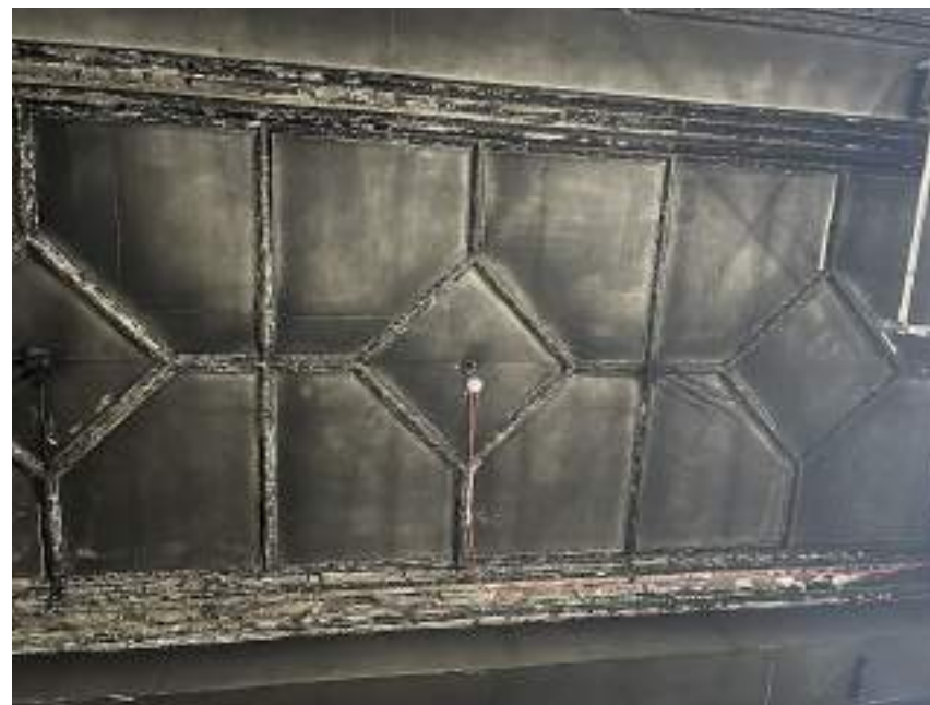
Figure 16: detail of the fire damaged ceiling taken on the day of sampling.
