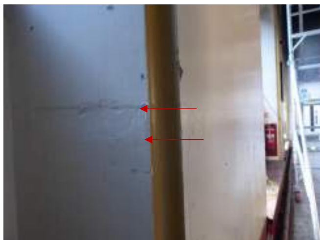
Figure 15: west elevation window reveal showing an apparent break in the underlying paint films.
