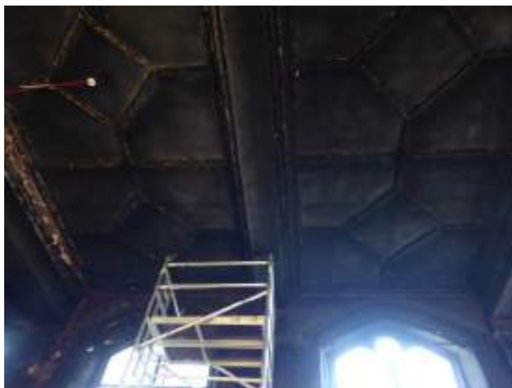
Figure 13: The blackened ceiling to the west side of Whiteley Hall.
