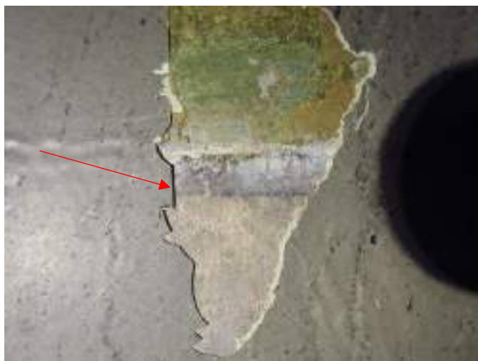
Figure 36: detail of upper wall paint exposure where pencil lines are seen in the void where a timber baton has been removed.
