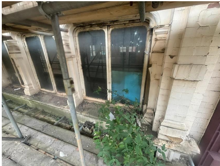
Example no. 8 – photo above showing second floor right hand lower windows Overall average condition showing flaking paintwork, weathering and vegetation growth.
