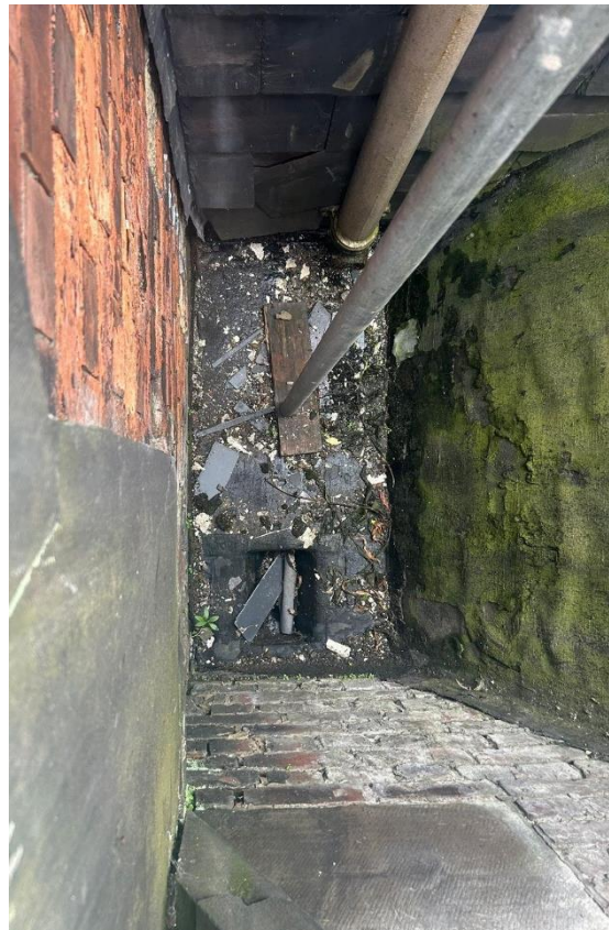
Example no. 10 – photo above showing rainwater outlets at parapet roof level Overall poor condition showing blown brickwork to other side of parapet wall, weathering and blocked rainwater roof outlet.
