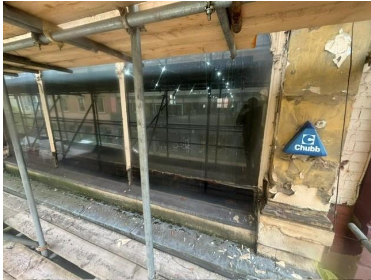
Example no. 9 – photo above showing first floor right hand lower windows Overall poor condition showing rotten timber window mullions.
