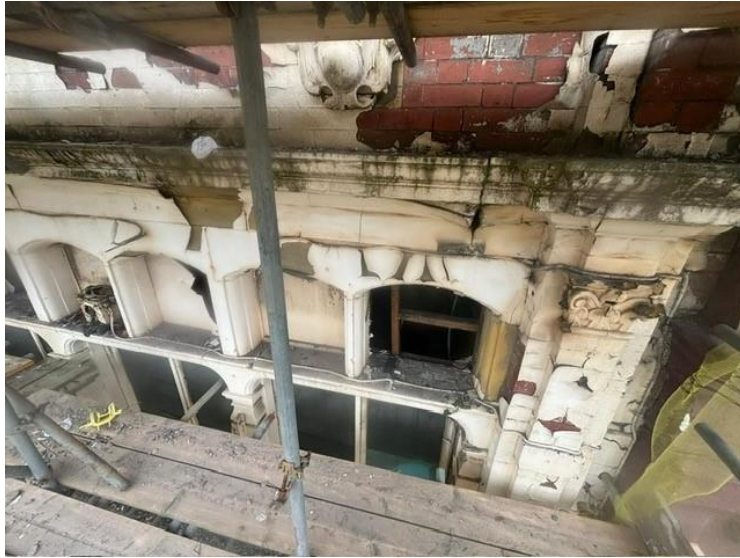
Example no. 7 – photo above showing second floor right hand upper windows Overall poor condition showing flaking paintwork, weathering and severe crack in stone cornice feature.
