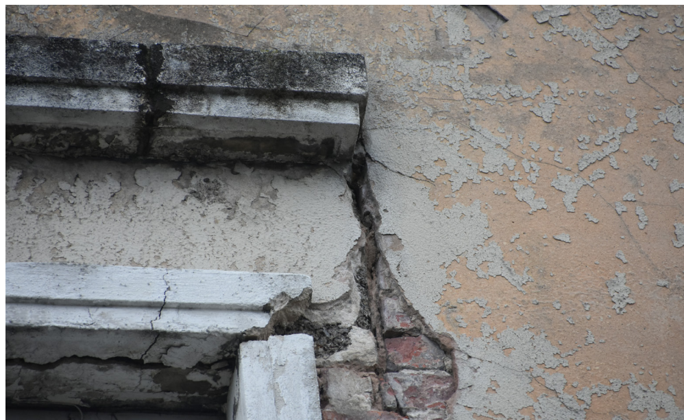
Image: Example of historic fabric in poor condition, surrounding window opening.
