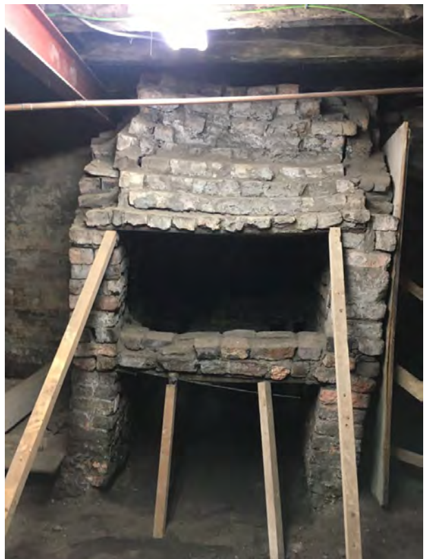
Fig.4 Basement oven being propped up due to unstable nature.
