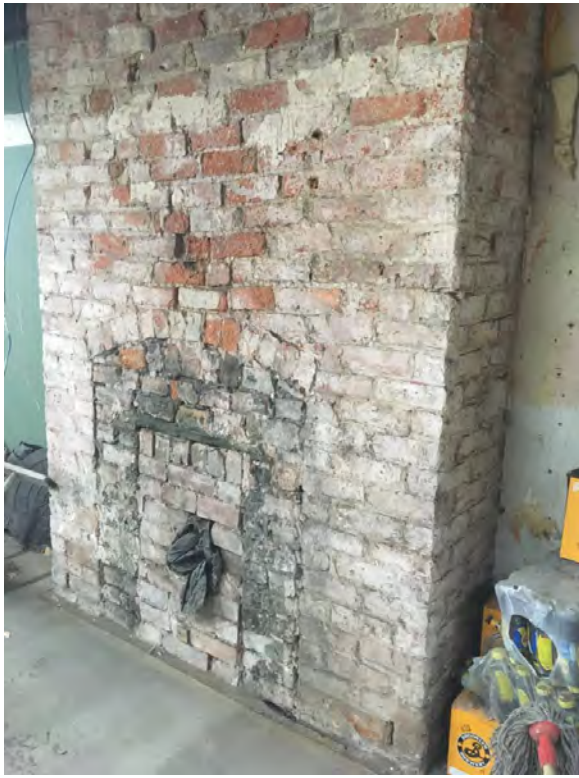
Fig 11. Front Fireplace modern plaster removed
