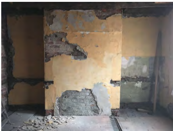
Fig 22. Front Fireplace, very loose plaster.
