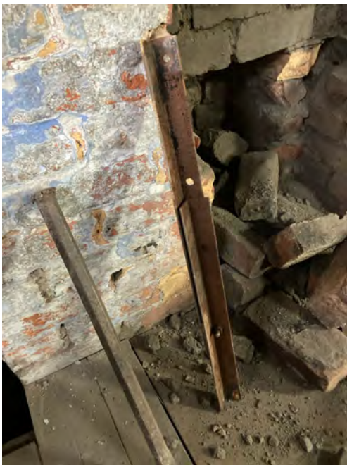
Fig 27. Angle iron from rear fireplace.
