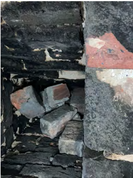
Fig 31. Photo of inside chimney of front fireplace filled with bricks
