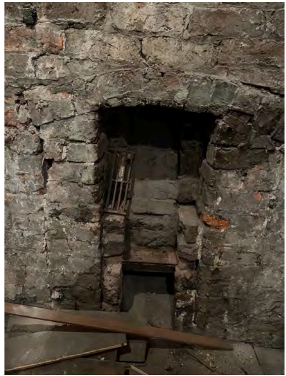
Fig 21. Rear fireplace opened to reveal broken iron grate.
