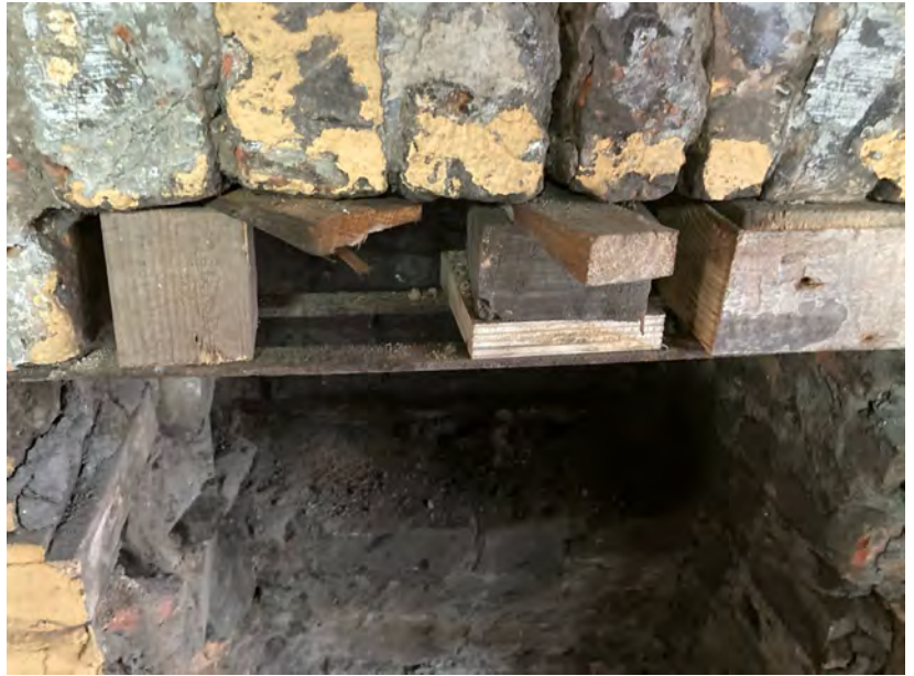
Fig 30. The brick arch steadied with timber packers as it was in a delicate state. Repair required.
