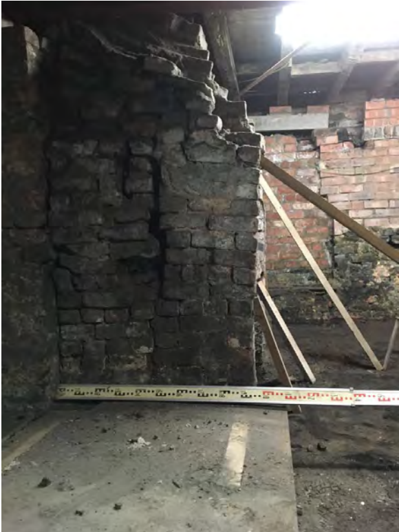
Fig 5. Side of Basement oven showing large fissure and movement away from the structure.
