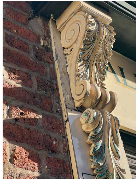
Fig 18. Close up of moulding revealed it was stuck onto new signage and not original.
