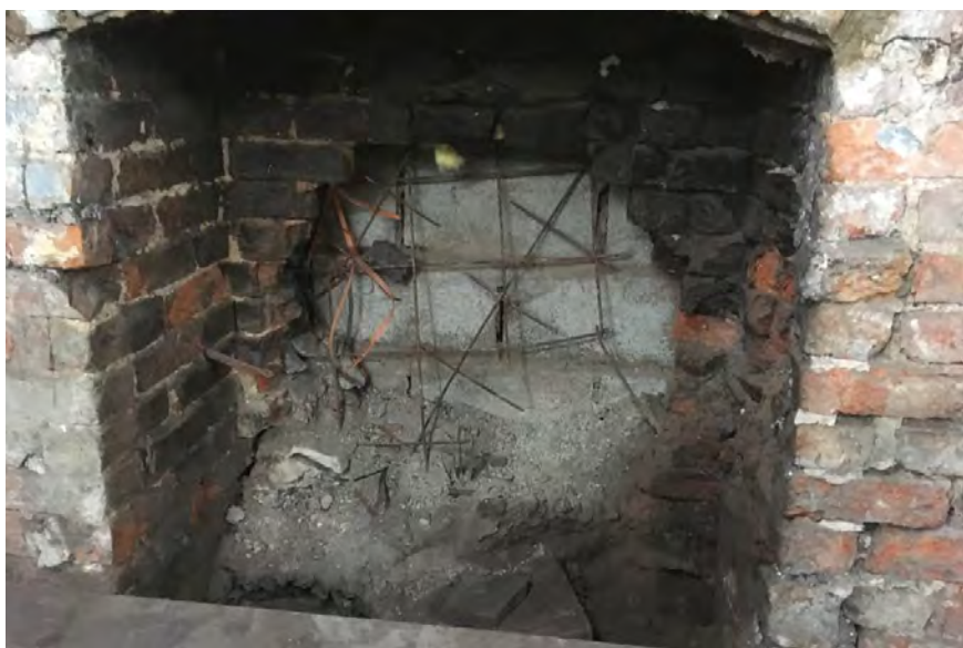
Fig 10. Back of rear fireplace showing broken chimney and breeze block work from The Bay Horse Public house.
