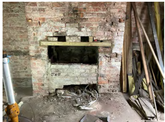
Fig 23. Removal of plaster revealed missing lintel, temporary one put in place for support.
