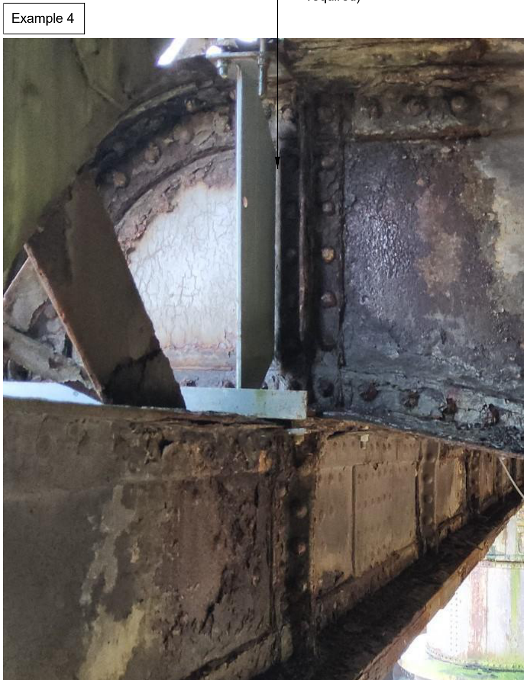
Air gap between stiffener and web plate - not as per 2022 detail which showed contact required)
