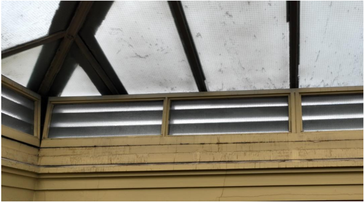
Fig 3. Current roof lantern, showing failure of louvres frame and water ingress. Photo by Robertson Group Ltd. 2024.
