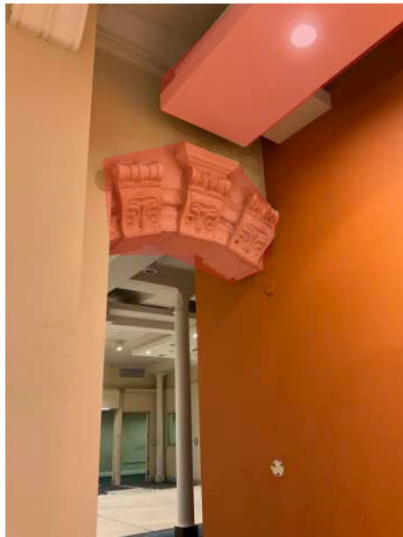
NON ORIGINAL FIXTURE WITHOUT HISTORICAL VALUE TO BE REMOVED
