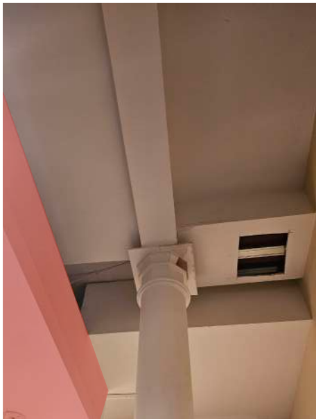
EXISTING EXPOSED COLUMN HEAD IN POOR CONDITION. CEILING RAFTS TO BE DEMOLISHED.
